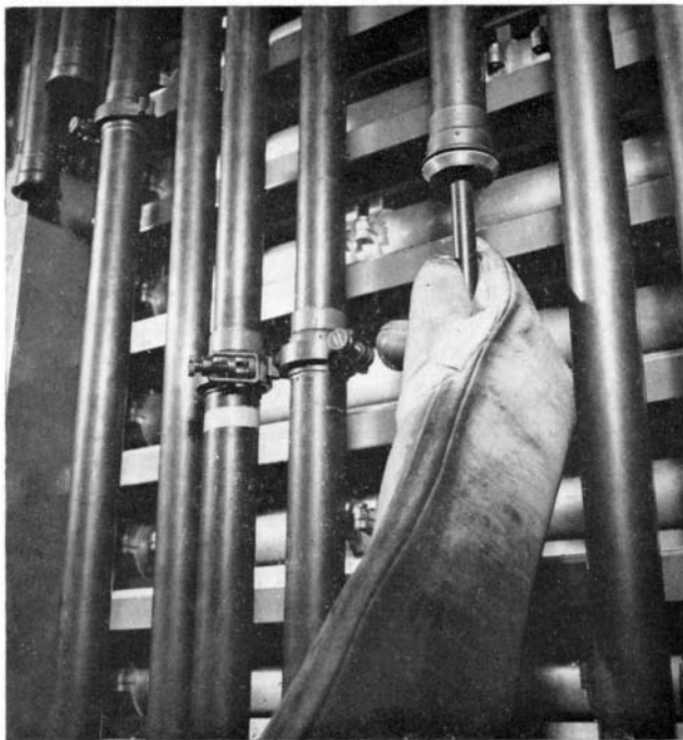
“Earthing the coaxial inner to prevent dangerous pick-up”
