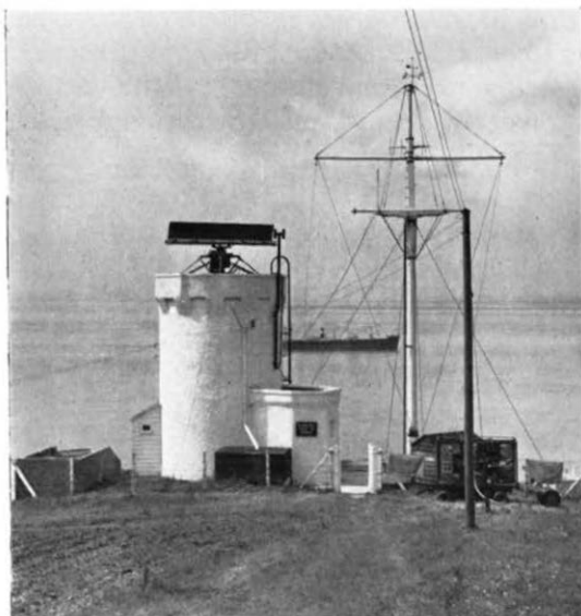
Marconi's new surveillance radar equipment mounted on a tower overlooking the sea; the transmitting and receiving aerials are on the adjacent pole mast
