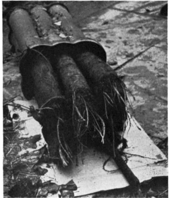
Tree roots in duct
