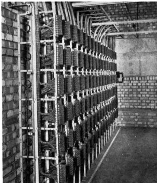
Main frame serving part of Plantation House, a large building recently completed in Mincing Lane
