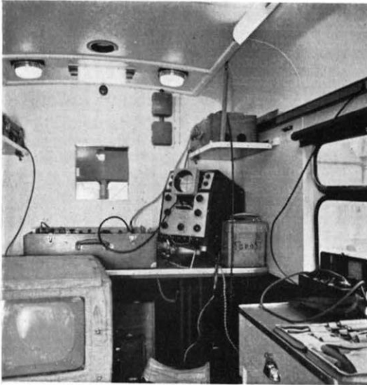
Fig. 2: Mobile repeater station—internal view showing video repeater equipment
