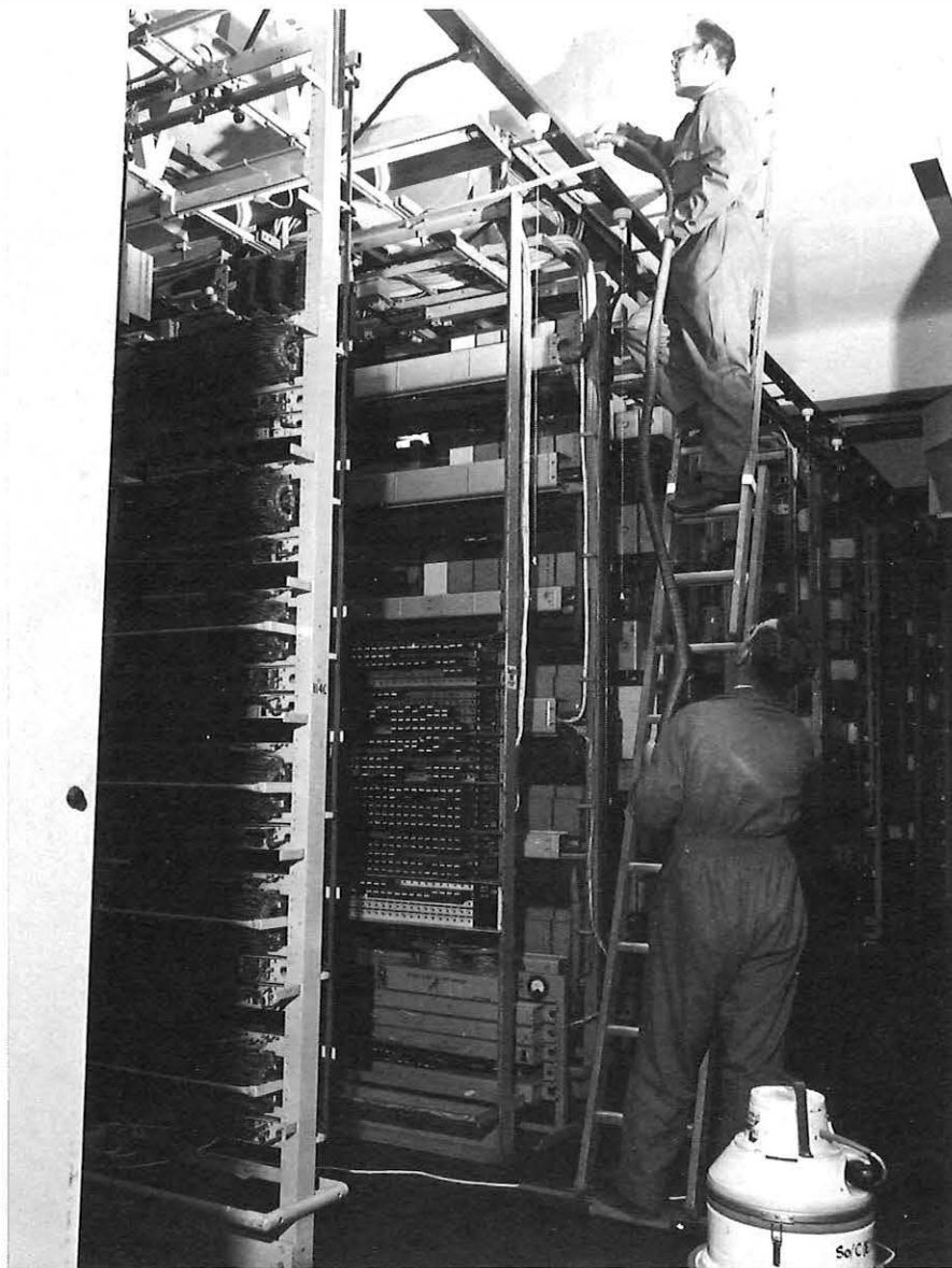
A mobile cleaning team at work on overhead cable runways at a South London exchange.
