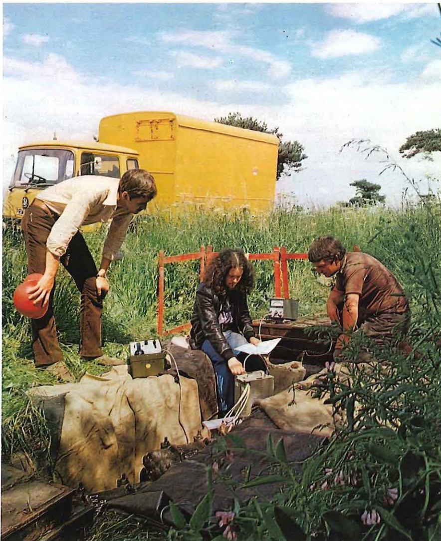
Coventry Area data transmission 'clerk of works' Dave Salter attends to maintenance of a buried footpath repeater on the Coventry-Northampton digital link. Maintenance joiners Malcolm Boston (left) and Richard Ramsay take a keen interest.
