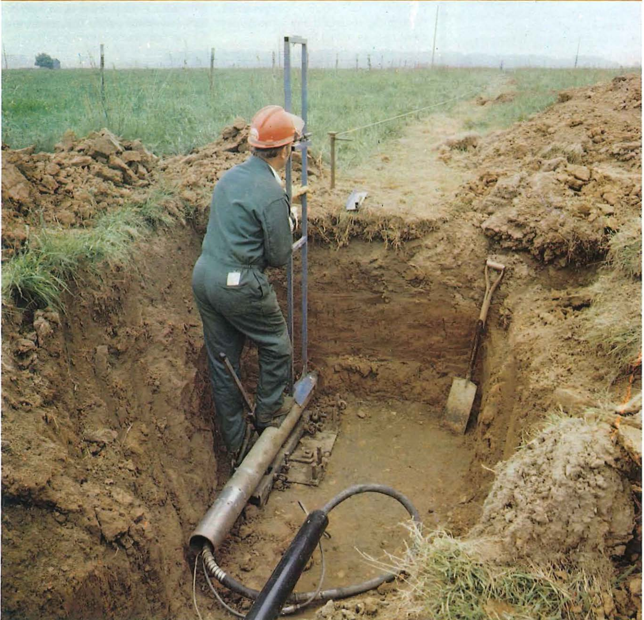
Engineering Instructor Mick Moore from Bletchley makes a telescopic sighting to ensure accuracy before the thrustborer is launched. This is the 130 mm machine.
