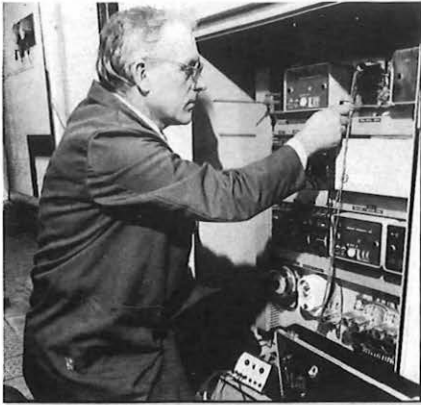
Energy 'troubleshooter' Trevor Woodyer checks motorised diverting valves used to heat a new apparatus room at Ascot Exchange using testers he designed and built himself.
