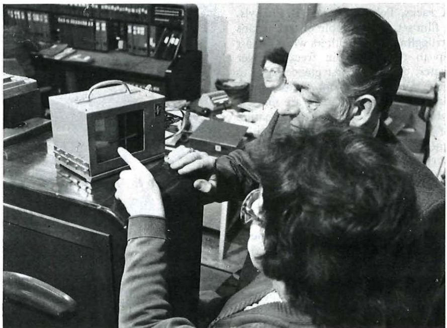
Fuel economy officer Roger Underhill and Ascot Acting Chief Supervisor Mrs Lillian Farmer check the temperature in the switchroom. The thermograph can also be used to monitor the effect of any economy measures.
