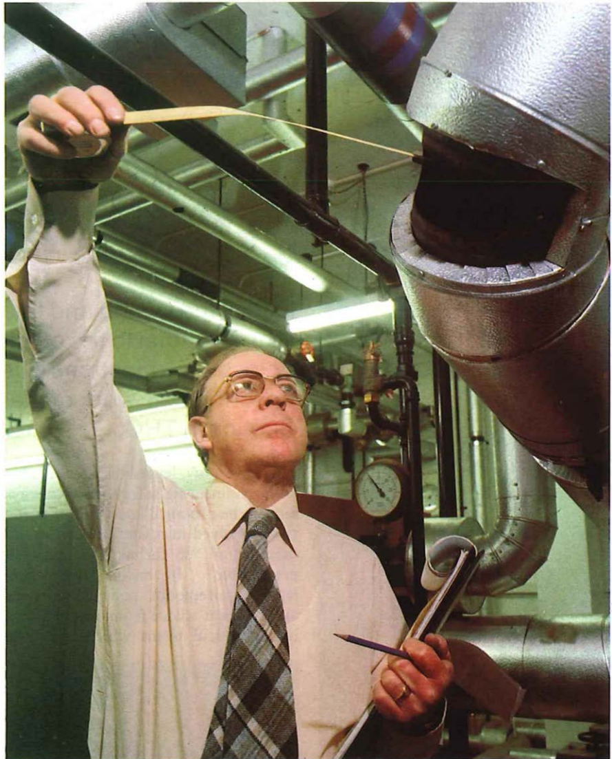
Roger Merry, fuel economy officer (accommodation), checks the diameter of an undersized outlet/flue on the main boiler at Ascot Exchange. The undersizing caused seals leading from the boiler to the flue to suffer pressure damage.
