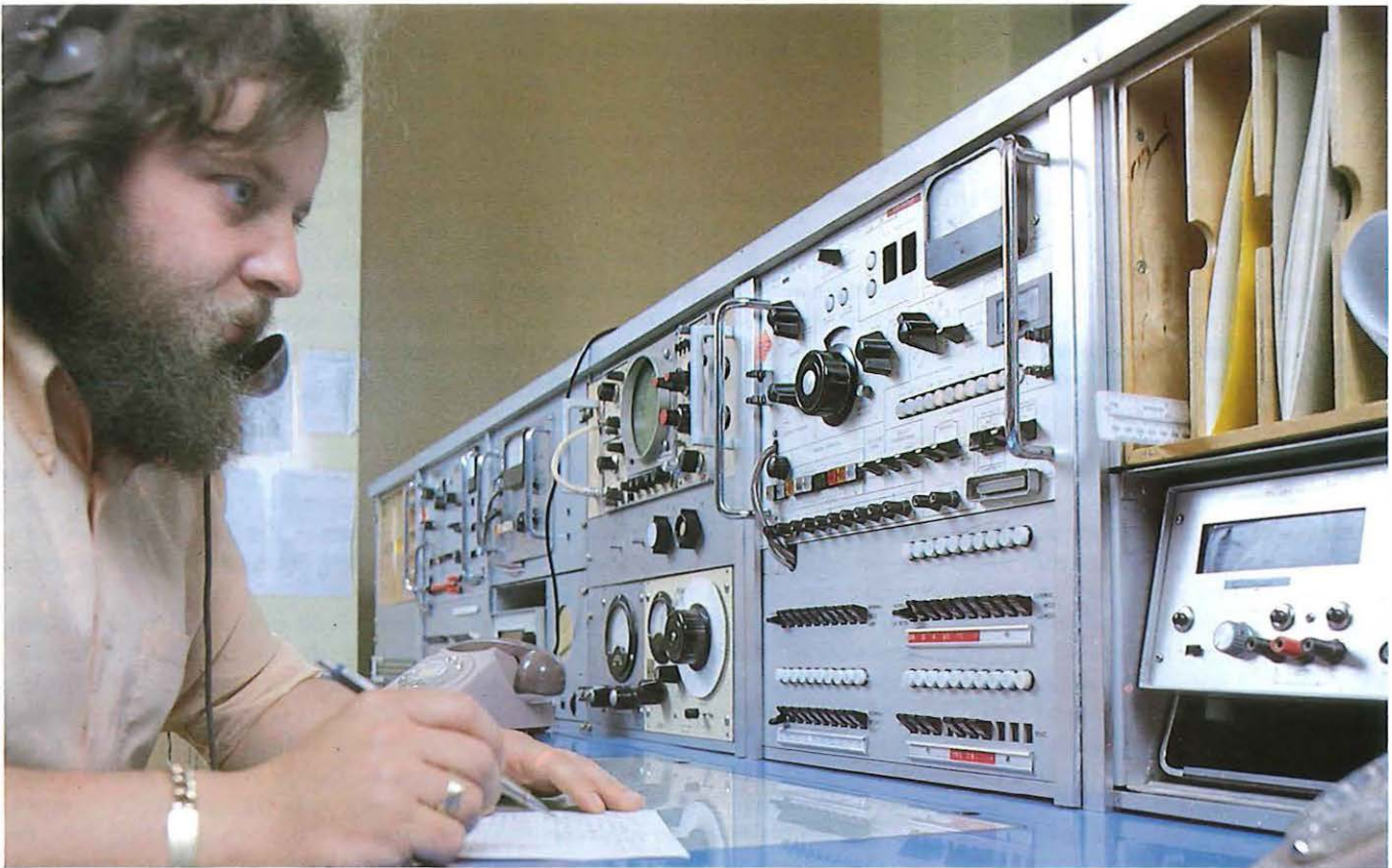
Technical Officer Ian Smith verifies a customer fault report at the London Datel Test Centre.
