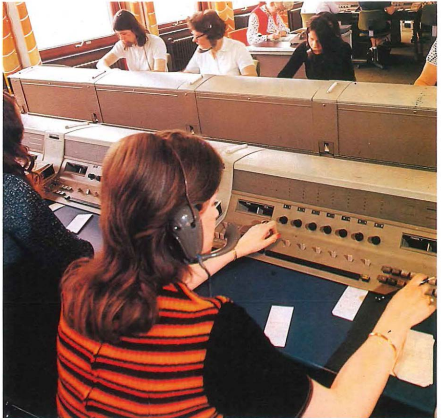
Operators at work on cordless switchboards of the type which have been installed at exchanges throughout the country in recent years.
