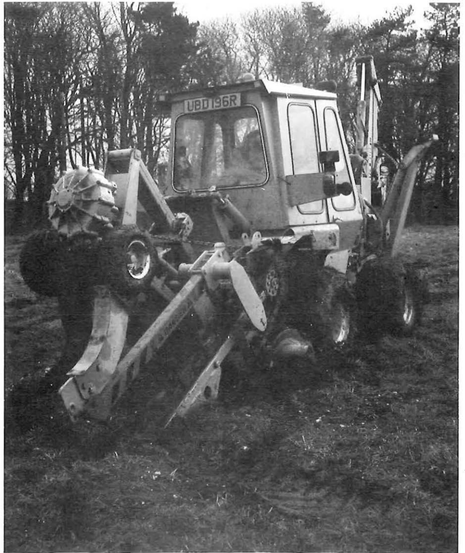
The chain type excavator at the back of the machine removes spoil prior to cable being laid in.
