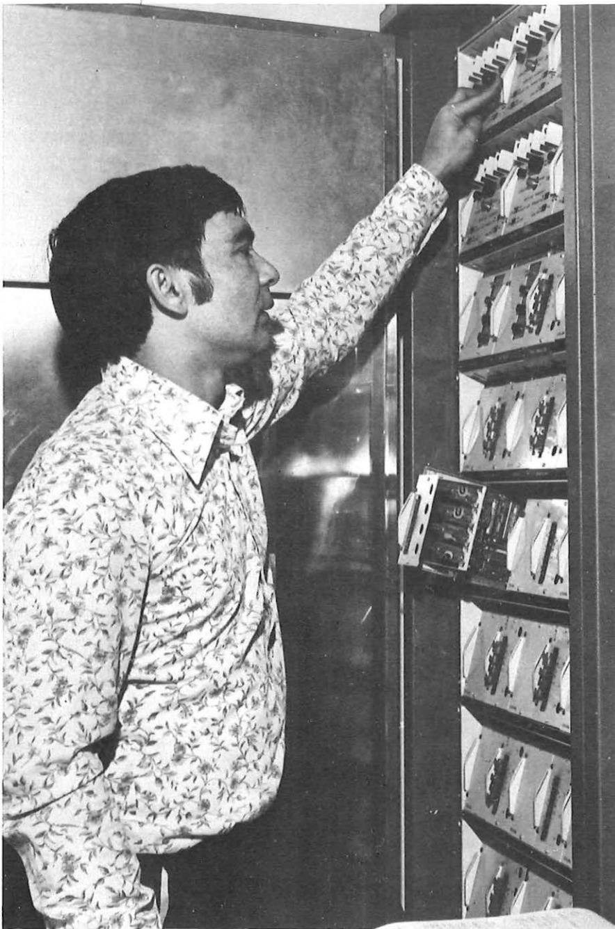
Technician Alan Grenouilland provides a new circuit on the broadcast and conference system which operates between the City offices of Lloyds of London and their Intelligence Department at Colchester.
