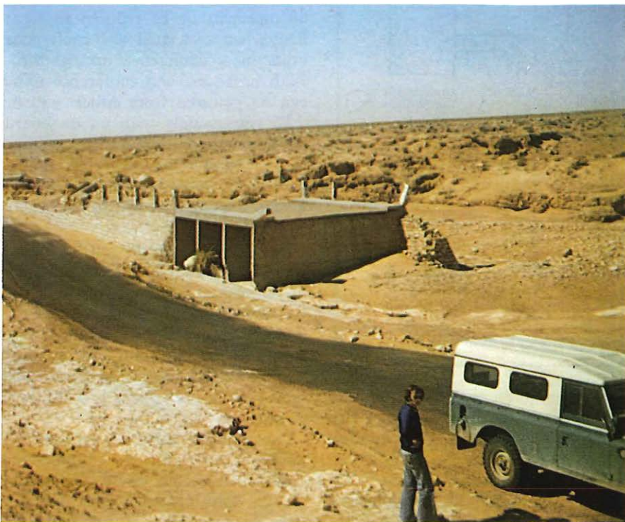
New development on the flood prone Qasr al Haj to Tigi road. A road bridge has already been installed and telecommunications cables must now be incorporated.
