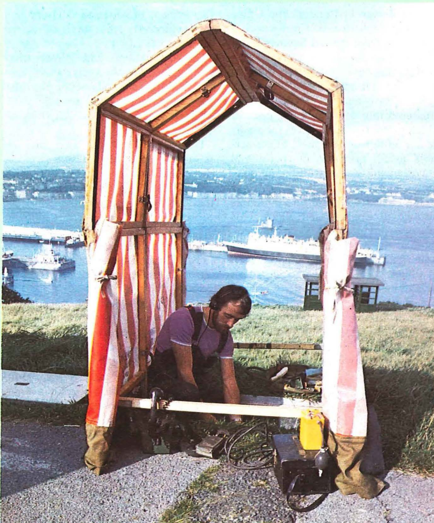
Technician Les Callow working on cables in a joint-box on Douglas Head, with the harbour and Douglas Bay in the background.
