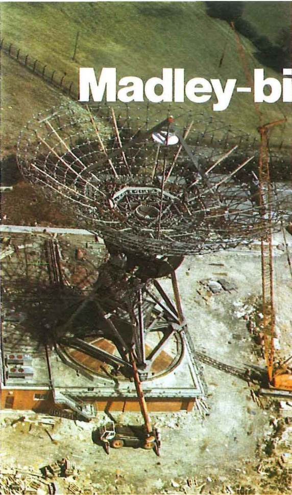
Construction work on the Madley 1 aerial dish shortly before the aluminium panels were lifted into position by crane.
