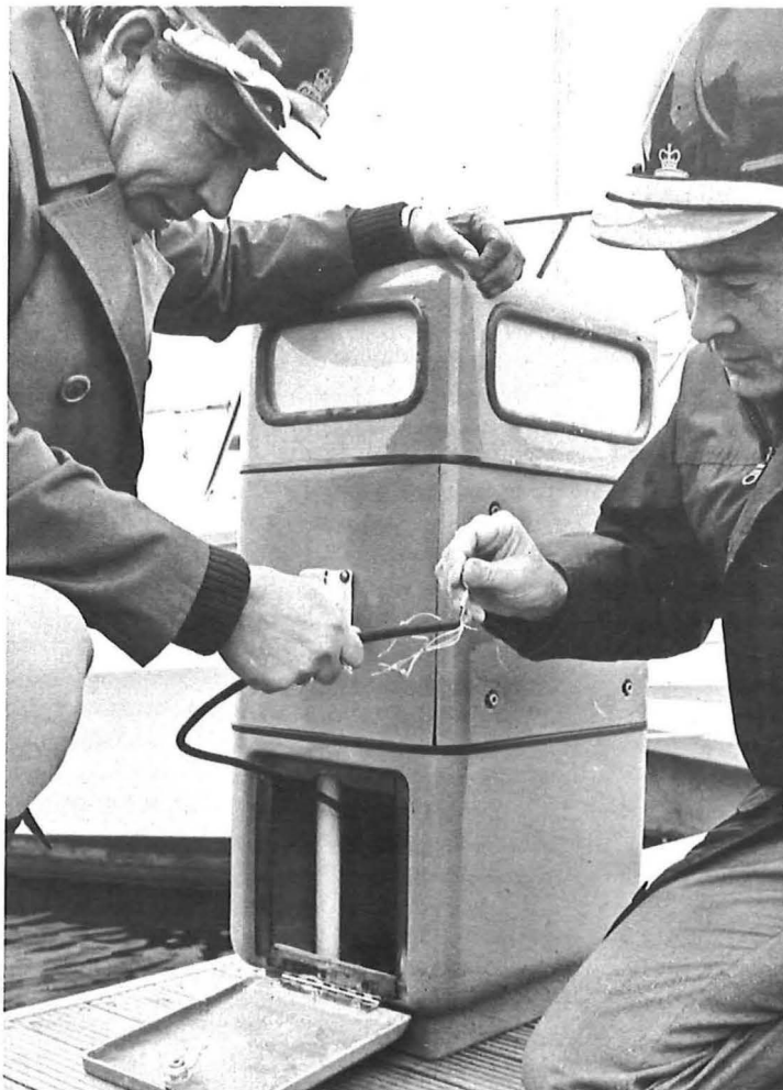
Co-author Mr George Evans and external maintenance engineer John Woodford provide a termination on the telephone cable serving one of the bollards.
