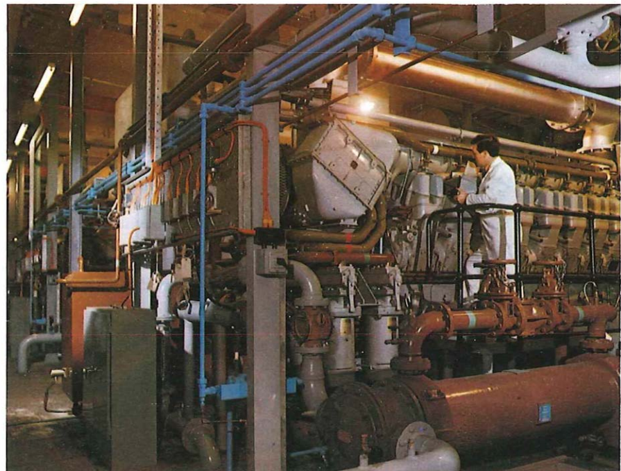
A contractor's engineer checks over one of the huge 45 ton standby engine sets which will come to life should normal power supplies fail.
