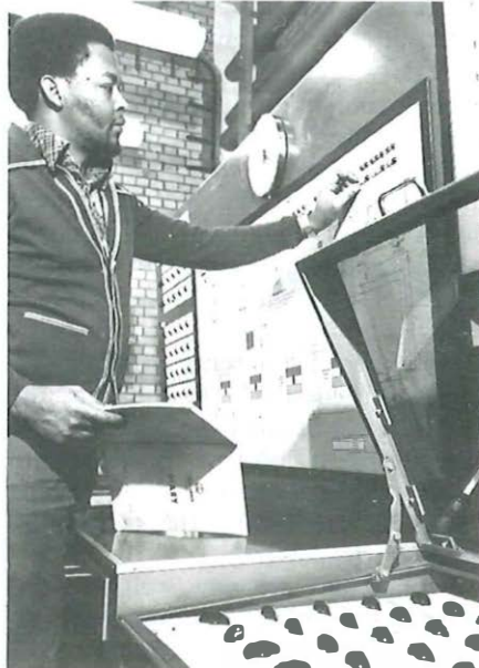
George Wright takes a reading at the engineering control centre where alarms from the various plants throughout Mondial are monitored.
