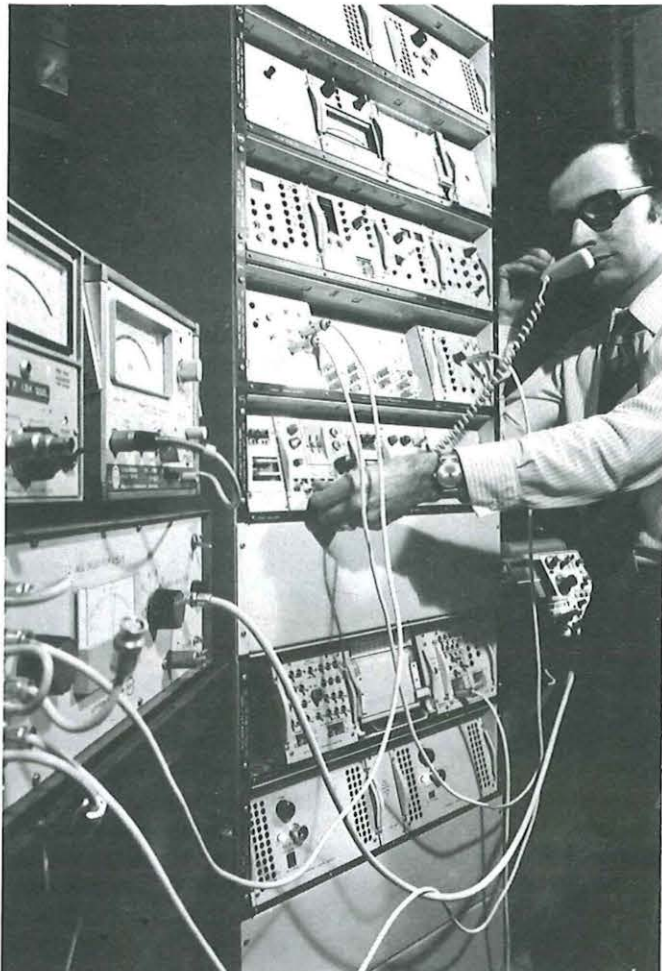
An engineer tests the terminal equipment of a high speed digital transmission system at a repeater station.
