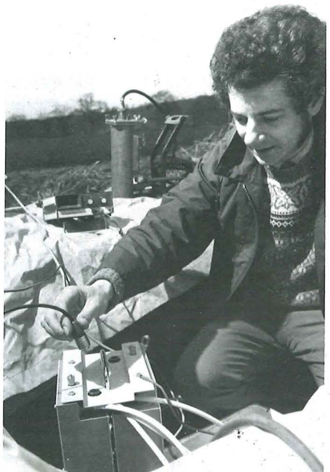
A roadside repeater installation is checked during work on the 120Mbit/s digital transmission system at Guildford.
