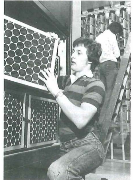
Technician Danny Smith prepares to change a filter in one of the building's air handling units. In the background Dave Fewkes, a Technical Officer works on an independent distribution frame.
