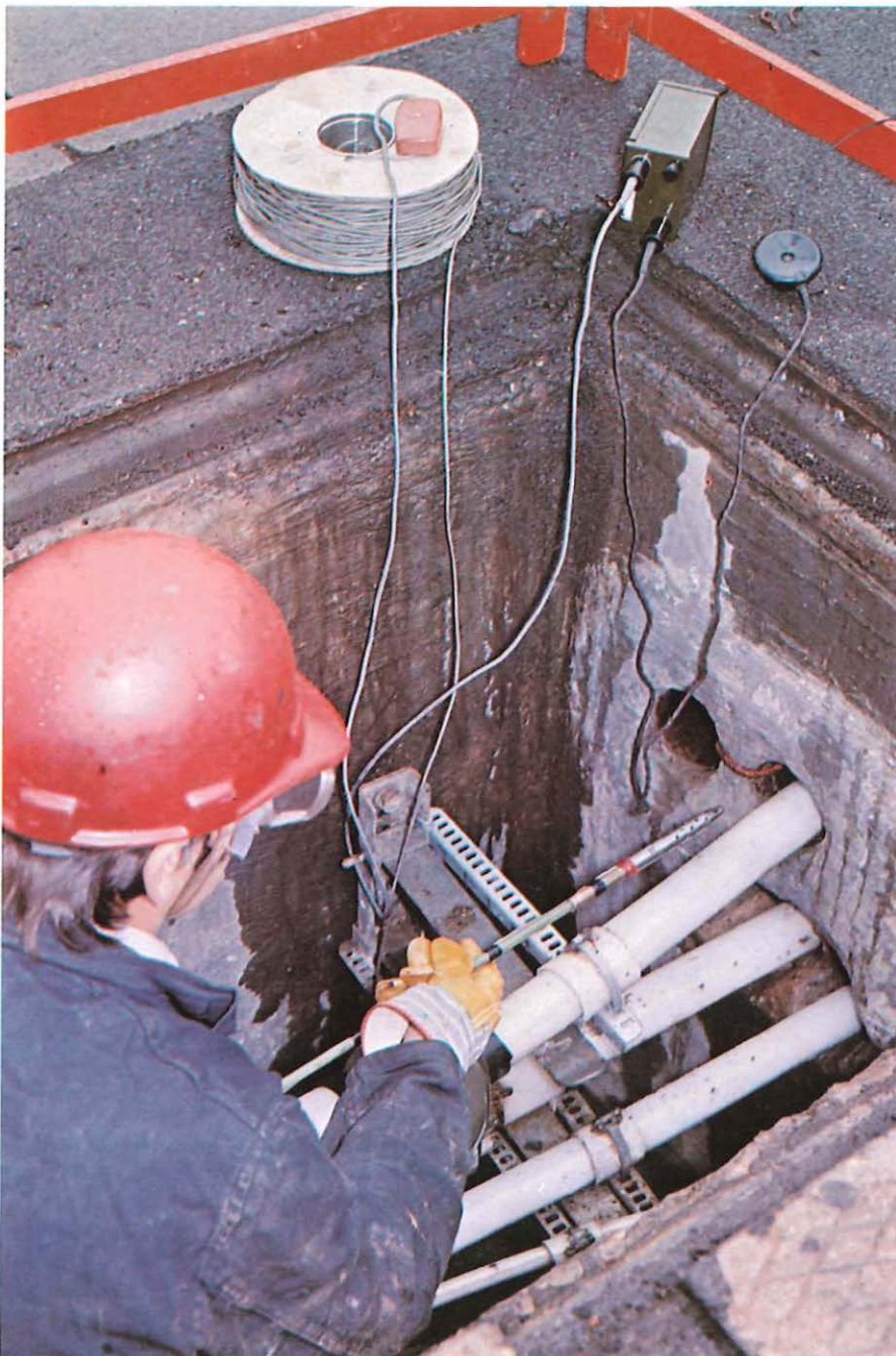
Technician Albert Wood inserts an audio probe into a duct to locate an air leak in a pressurised cable between two jointing access points.
