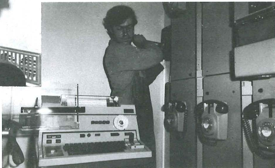
Below: Mr Neil Smith from Guildford workshops fits the terminal block in the unit's storeroom. The alternative wallboards and teleprinter can be seen.
