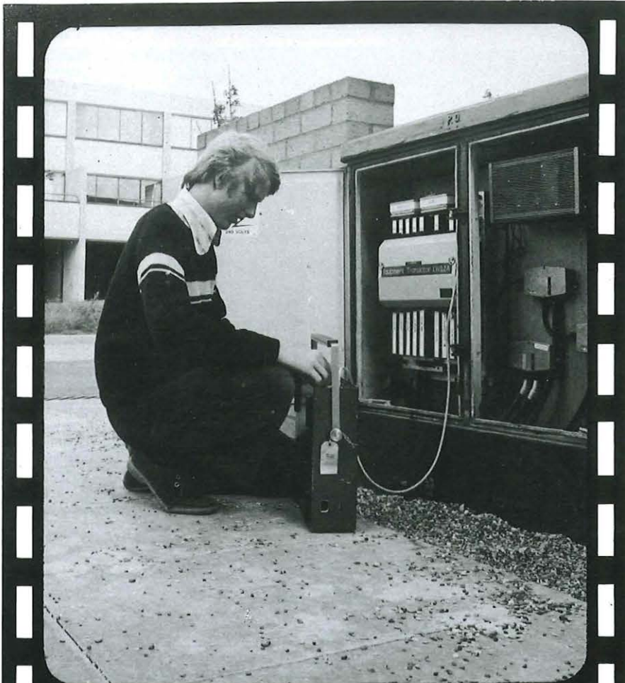
Left: Trainee Technician Apprentice John Simmons measures television signal levels on the VHF/UHF translator equipment at a roadside cabinet.
