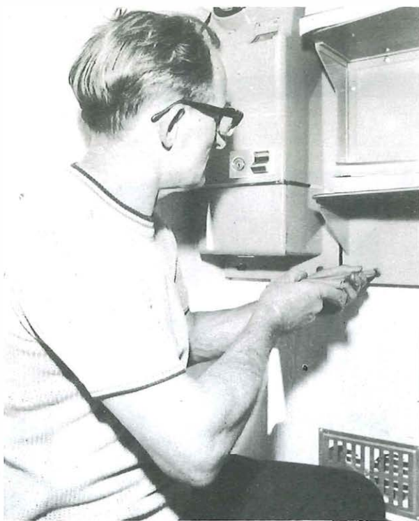
Left: In the new trailer unit, Technician Norman Hawkins prepares to remove a coinbox telephone from a 'kiosk' and replace it with a wall type non-coinbox telephone.
