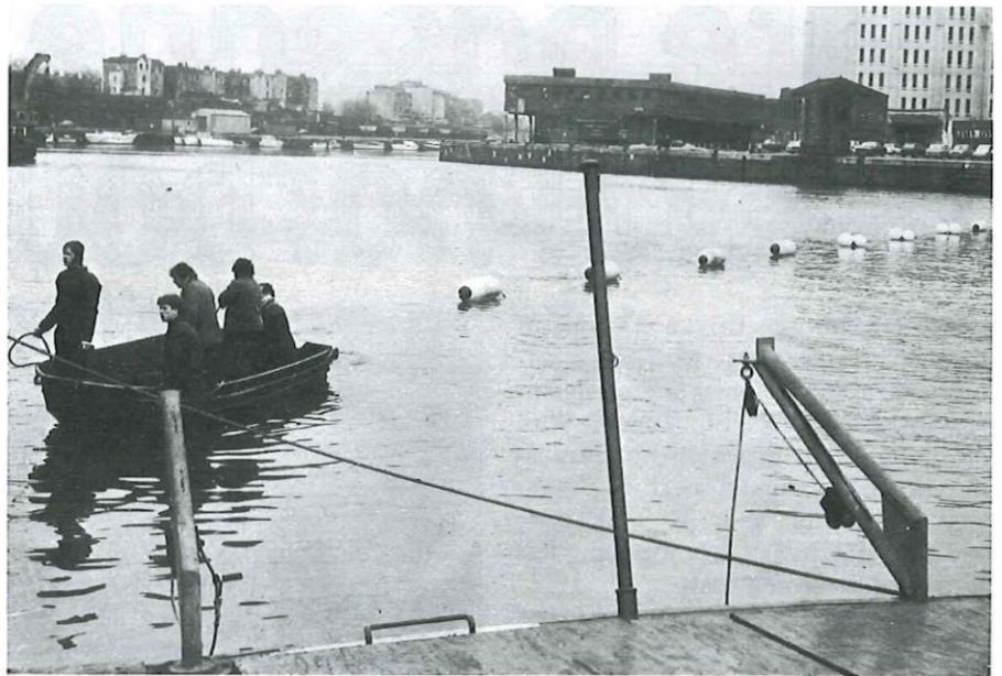
The first duct length being towed across the harbour from its assembly point.
