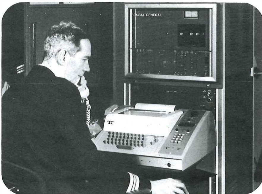
The Comsat General terminal in the liner's radio room, which provides facilities for telephone, telex, data and facsimile communications via satellite with international networks.
