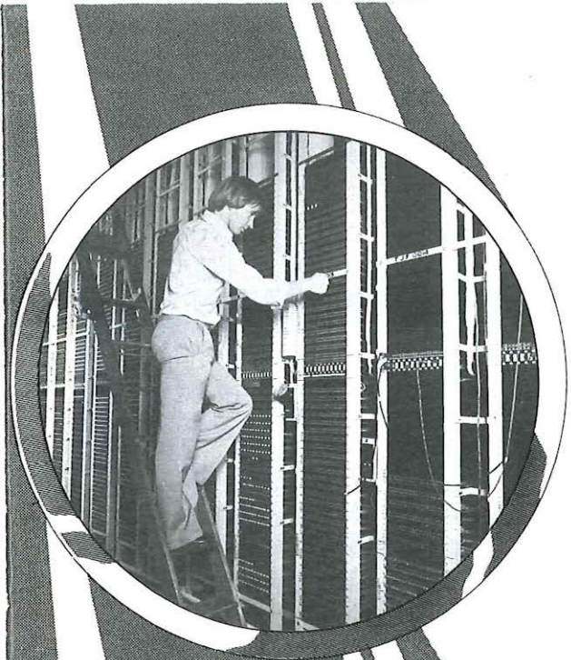
Technician Jed Isbell connects a circuit on the test jack frame at Cambridge TMCC.
