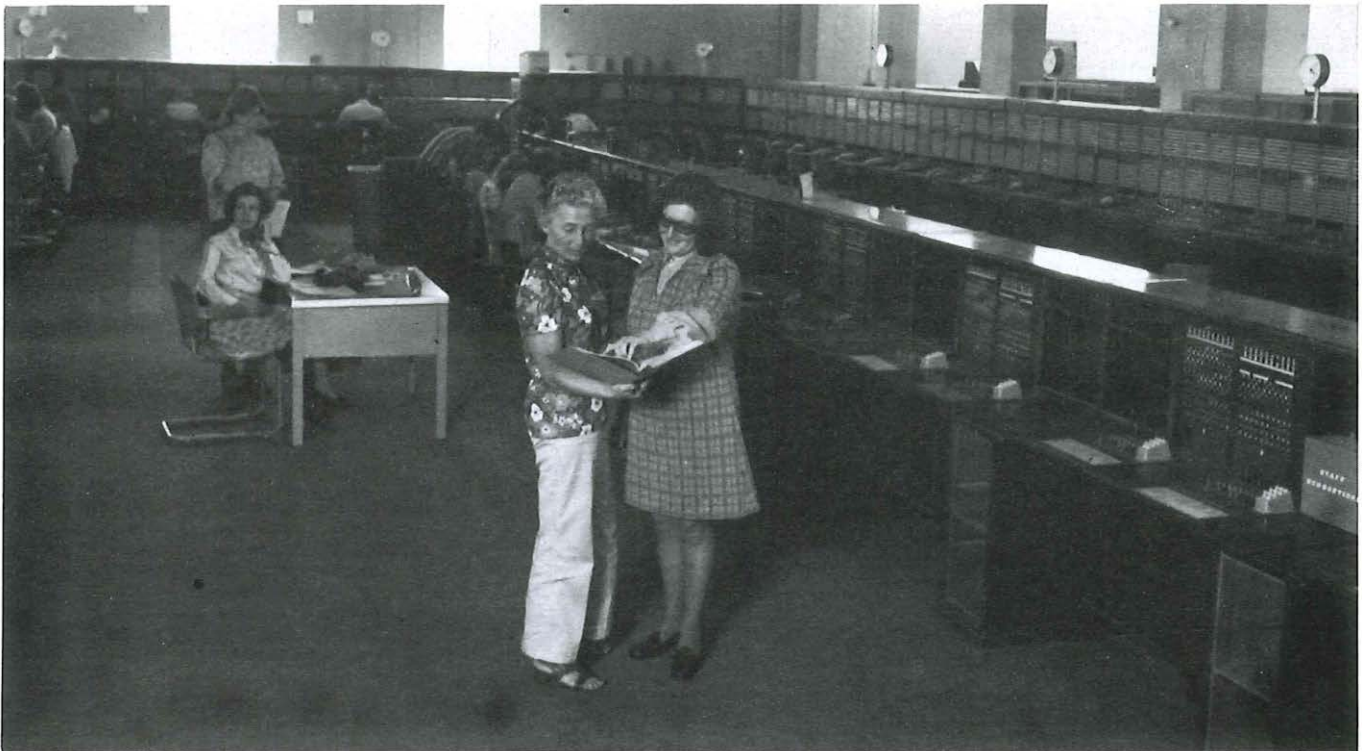
Typical older-type switchroom of a medium-sized Operator Service Centre, showing how relatively few fitted positions are now staffed. Enquiry positions are located down the centre of the room.
