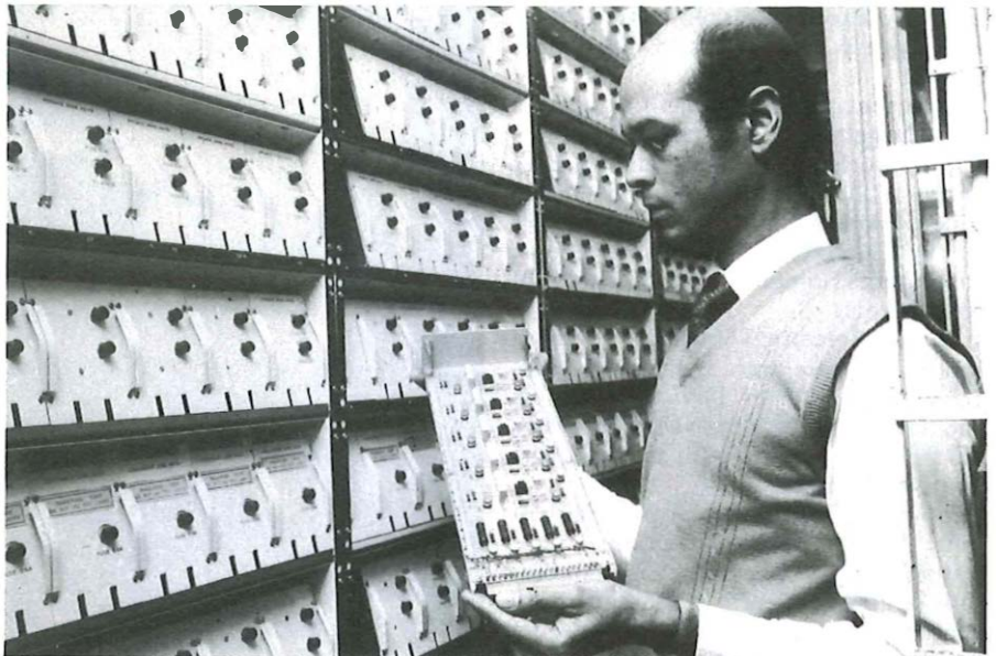
Post Office Technician Moreil Lacide examines a console control circuit in the apparatus room adjoining the dealer board installation.
