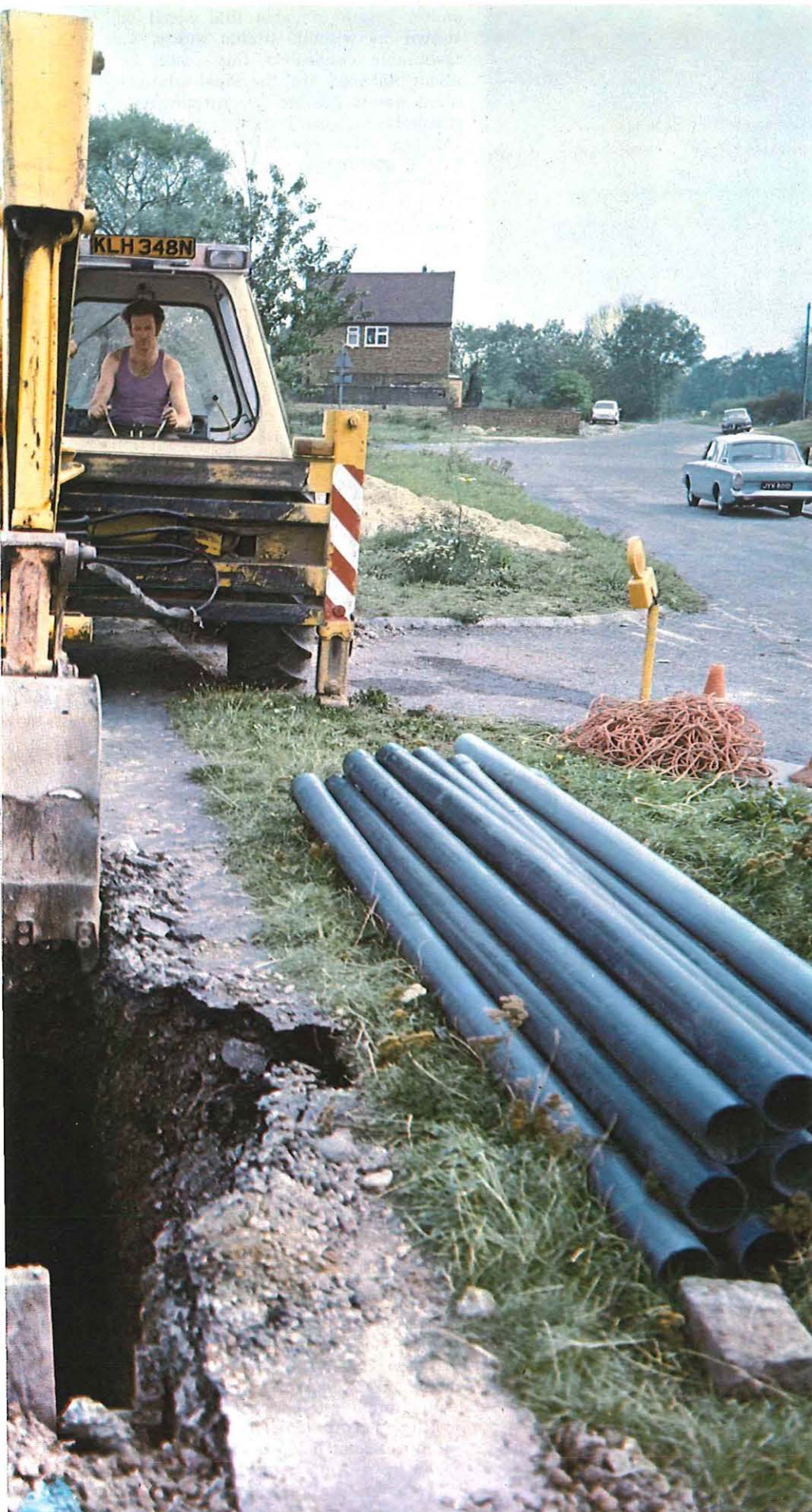
A mechanical digger channels out the final stretch of trenching necessary for the 60 MHz duct in north west London.
