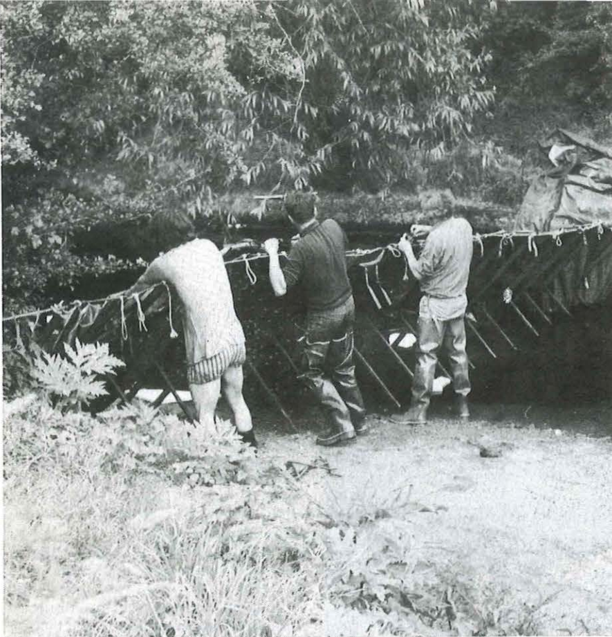
Above: A temporary dam had to be built across the River Brent in west London to allow the duct to be laid in a riverbed trench.
