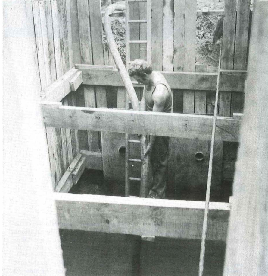
Water is pumped out of the last repeater manhole to be constructed along the route of the 60 MHz duct. The duct ends can be seen just above the water level.
