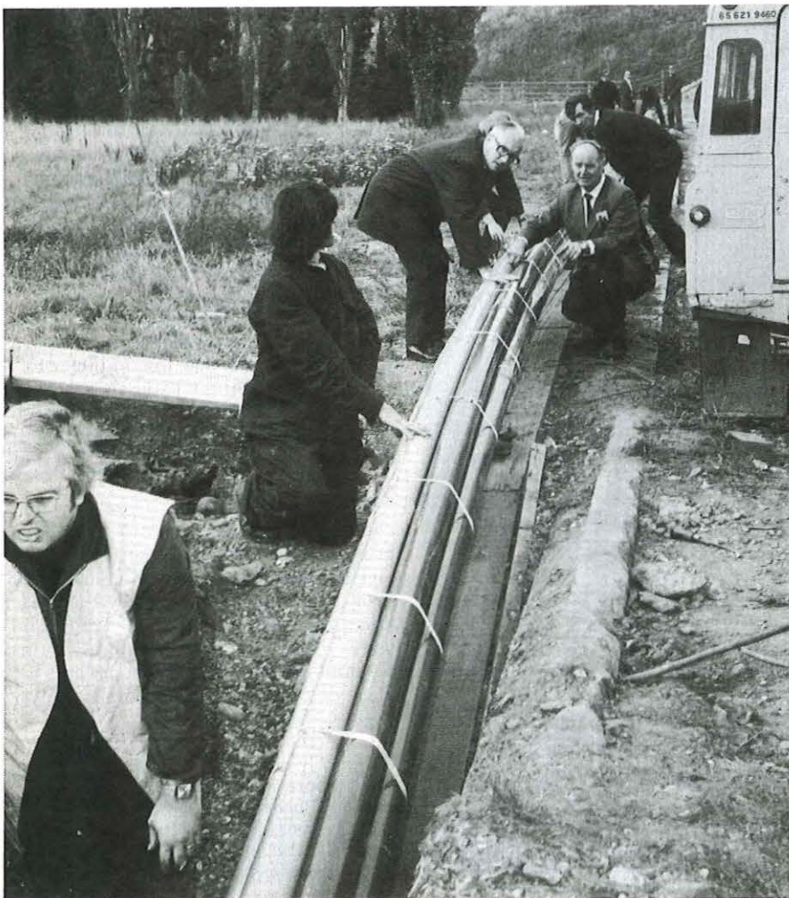
Below: At an Uxbridge roundabout the duct is prepared for its passage under the roundabout via a disused gas main.
