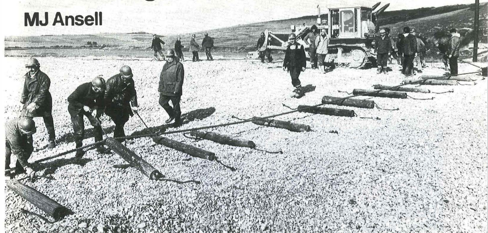
Poles are laid out on the beach at Cuckmere, near Eastbourne, to bring ashore the first high-capacity undersea telephone cable to be laid between France and Britain for 25 years. The cable came into service in September.
