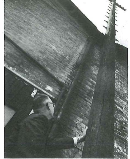
More than 70 years old and still going strong... the 1904 pole being examined here by Bryan Hambly, an inspector of major works in Bedford Telephone Area, carries lines at a local timber yard.
