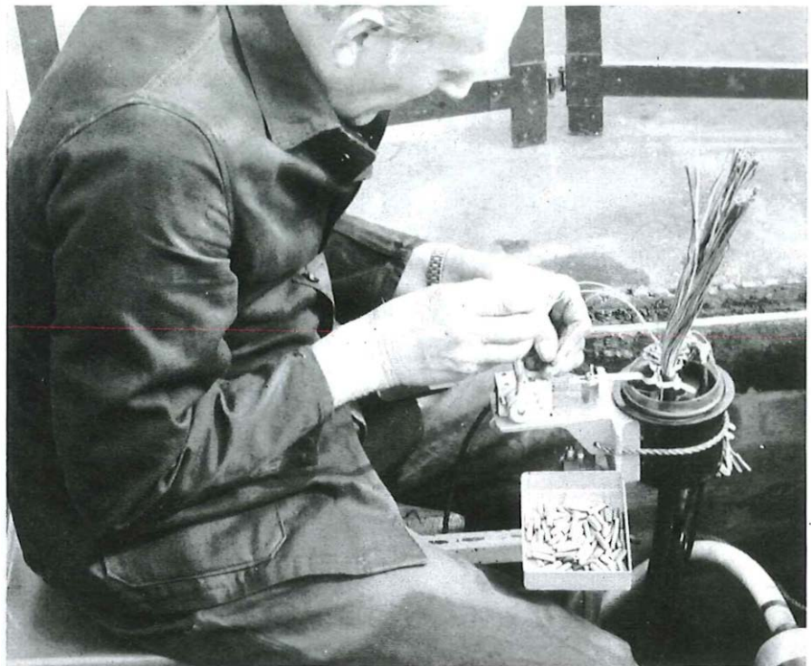
Above: This specially developed jig simplifies jointing of local distribution network cables. A cap-ended closure provides easy access to the jointed wires.
