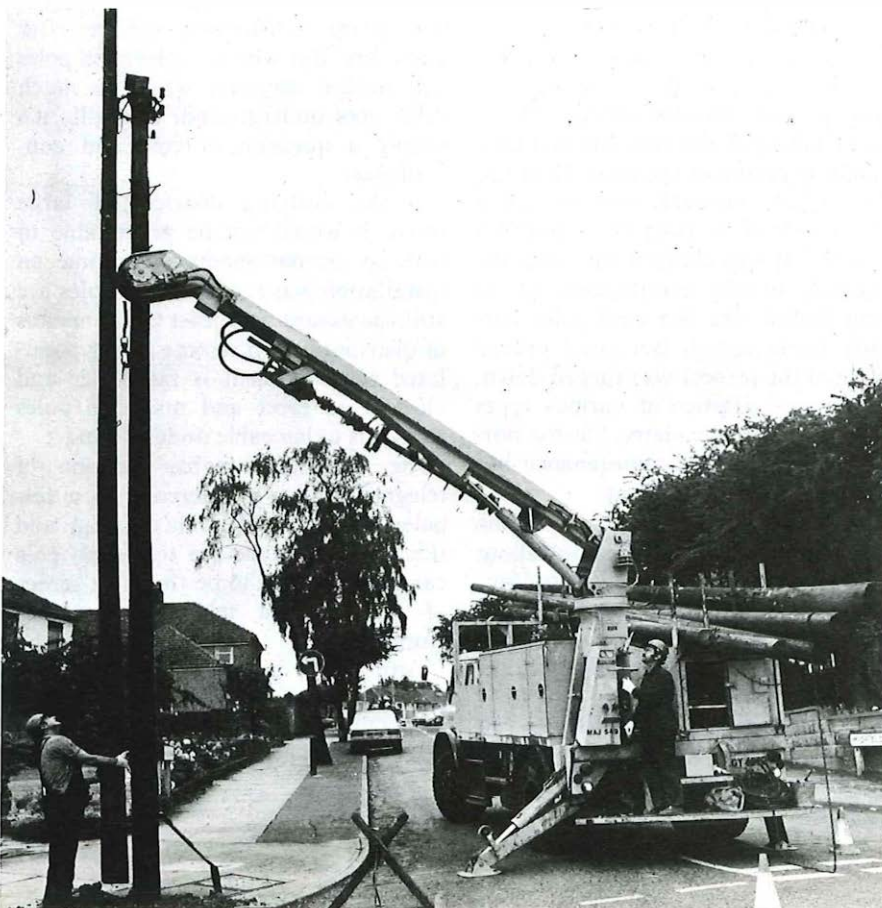
Post Office technicians Stan Andrews and Charlie MacLean erect a new pole alongside a decayed one, which will later be removed. On top of their vehicle is a pole which was replaced after giving nearly 80 years' service.
