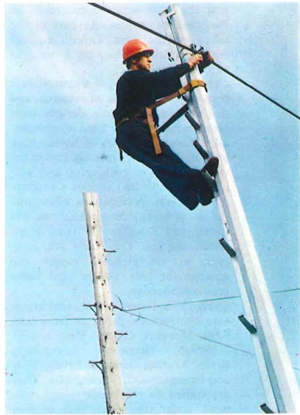
A galvanised steel pole undergoes tests alongside a more familiar wooden type at the Post Office's Smallford Test Centre in Hertfordshire.
