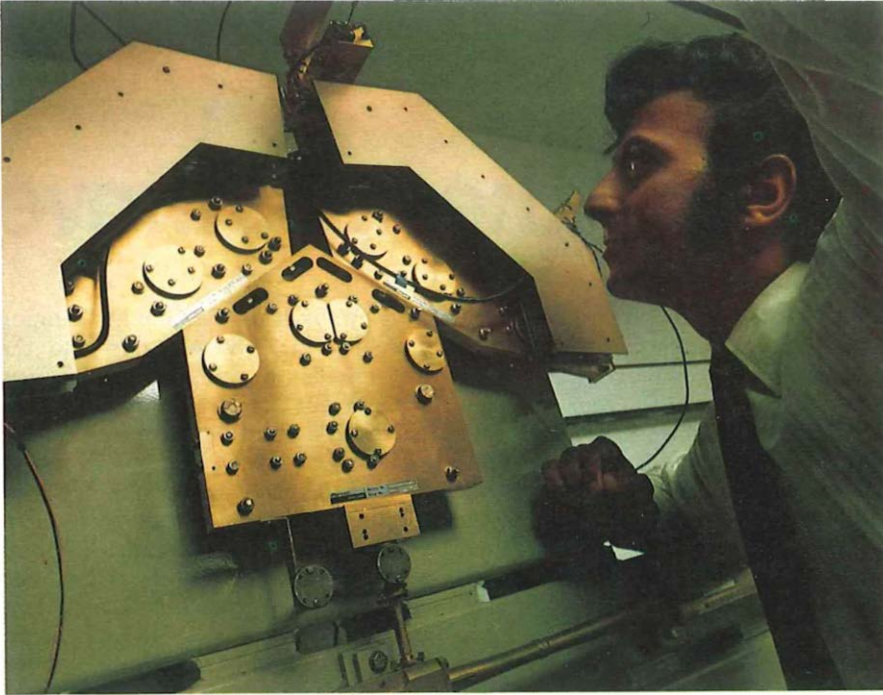
Post Office experiments on waveguide transmission systems could lead to more than 300,000 telephone circuits passing down a tube no bigger than a car exhaust. Here work is carried out on part of the terminal equipment of a 14-km waveguide system set up between Martlesham and Wickham Market.
