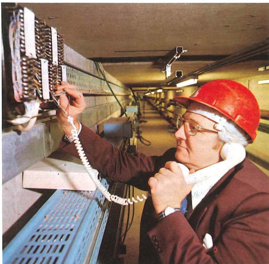
Telephone connections are checked in a service tunnel which runs underneath the exhibition halls.
