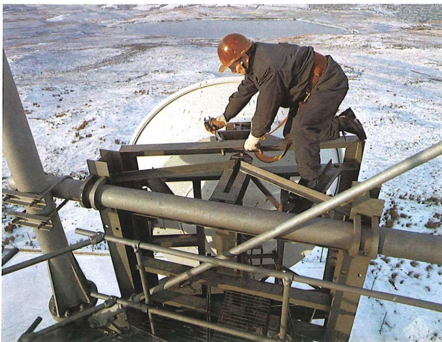
On a hill high above Greenock a Post Office engineer adjusts an aerial on one of the radio towers which form vital links in the Highlands and Islands telephone network.
