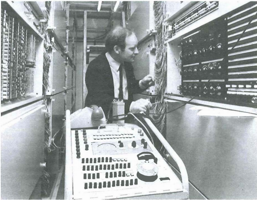
A check is carried out on a wiring block at the London main tandem switching centre in Unilever's private network.
