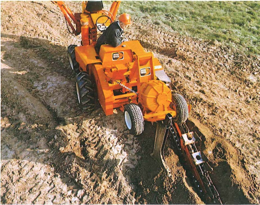
Known as the "Ditchwitch", this multi-purpose trench digger, moleplough and earth scooper undergoes evaluation trials at Smallford. Staff at the centre are proud that they can simulate most types of working situation.
