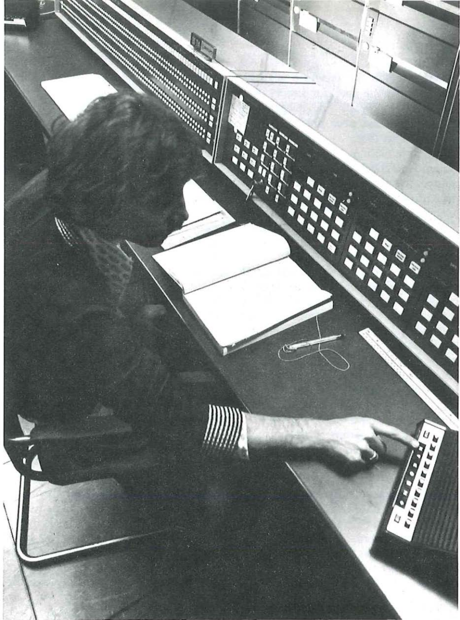
The technical control position at the TRC, from which operation of the computer system is supervised and controlled.
