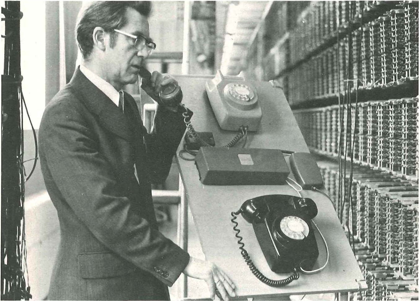
The audio line of a One plus One system is tested at Cardiff's main telephone exchange. The lower telephone is used for testing the carrier line.
