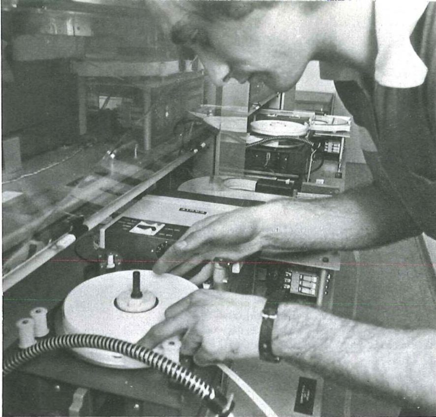
Each switching unit of an SSC has an equipment monitor. Here the tape is changed on one of a monitor's five paper tape units which record call failure reports.
