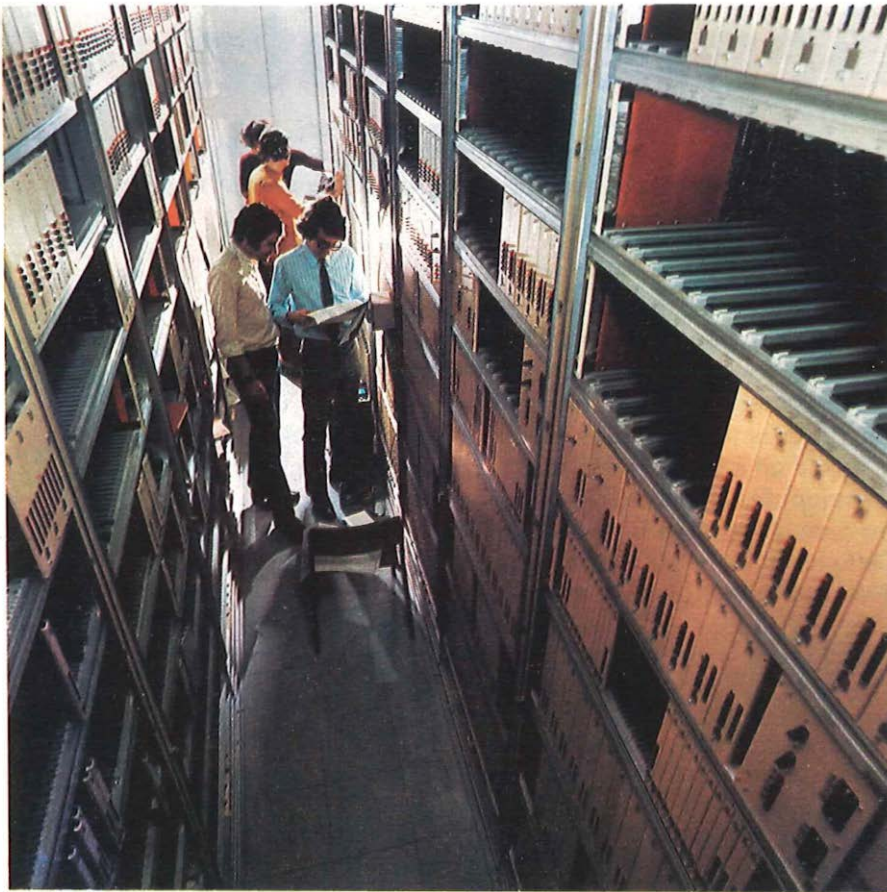
Installation and commissioning engineers work on a production TXE4 exchange at Rectory, near Birmingham.
