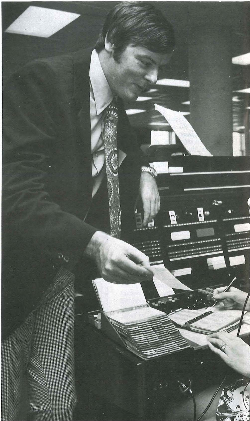
The author, formerly a superintendent at London's Shoreditch telephone exchange, is shown an operator's position on a cordless switchboard in Vancouver. "To my dismay, I was put on a switchboard after only an hour's training," she reported.
