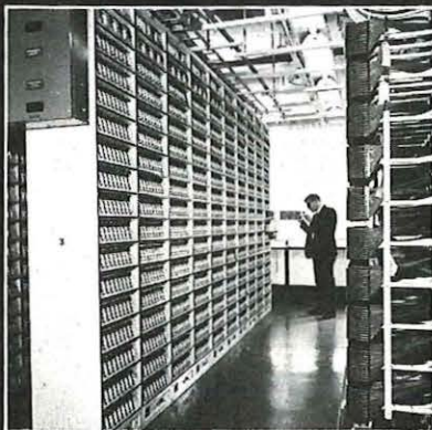
Telegraph Multiplex in London International Telex Exchange.
