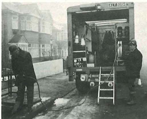
The rodding and light cabling vehicle is a self-contained unit used for laying cable in underground ducts. A crew member is pictured here in wintry conditions preparing equipment for pumping water from a jointing chamber. The pneumatic pump is connected by flexible pipe to an air compressor in the vehicle.
