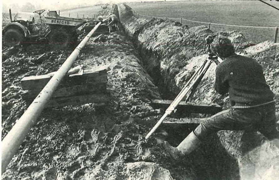
A tubular steel duct which will house the waveguide is being laid about four feet deep over the route of the trial. Here a surveyor checks the line of the trench while preparations are made to lower the four-inch diameter duct which has to be constructed with fine precision.
