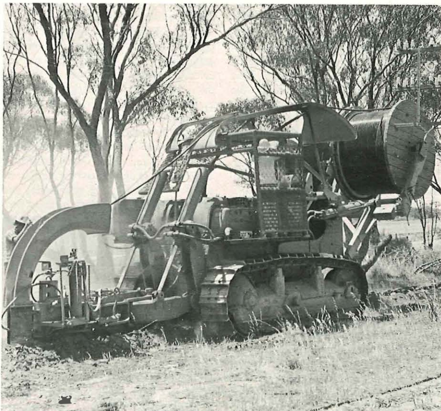
A cable layer in operation on the 1,140 mile Perth-Geraldton-Carnarvon coaxial cable project in Western Australia – one of the longest coaxial cable trunk system routes in the world.
