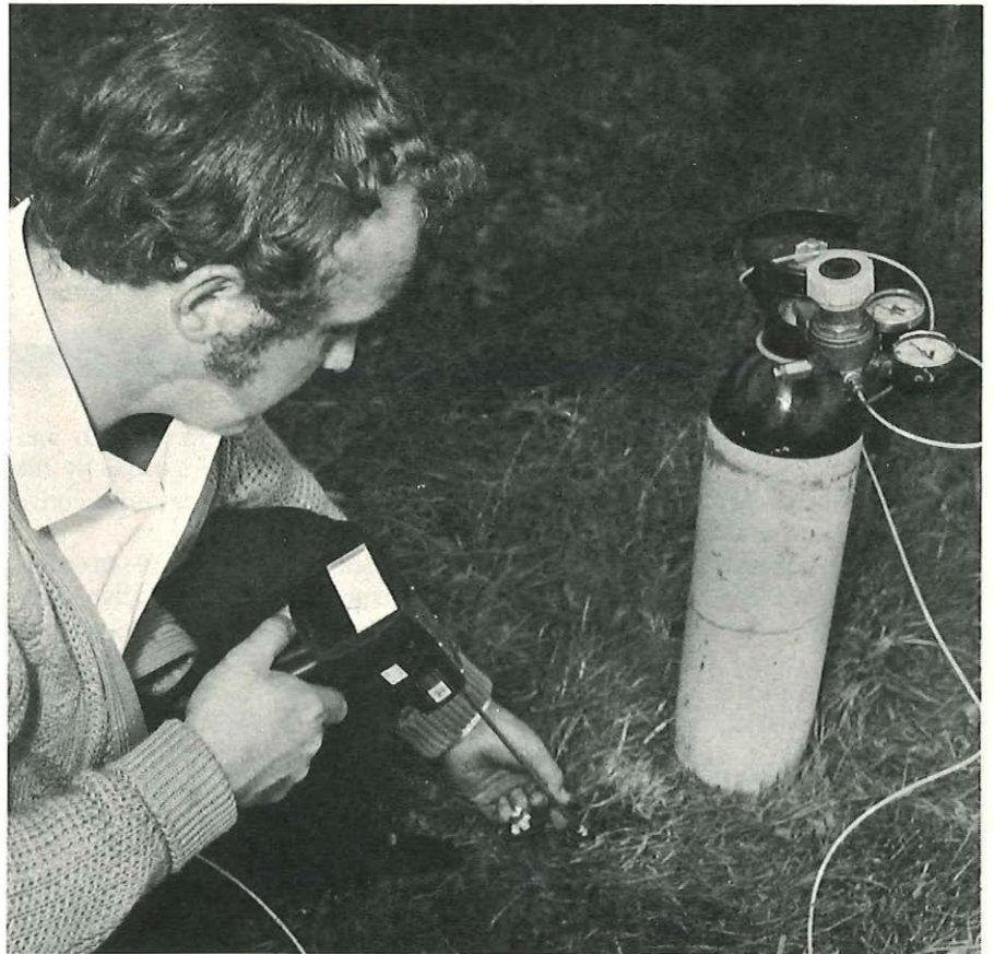
Technical Officer Eddie Belcher uses the detector to “sniff” for tracer gas at a hole bored directly above a cable which has been laid without duct. Any gas leaking from the cable would rise through the hole. Right: The detector “sniffs” for tracer gas at the outlet on the pump which is sucking air from a cable duct.
