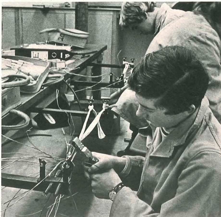
Right: Trainees learn polythene cable jointing in one of the training centre's work rooms.
