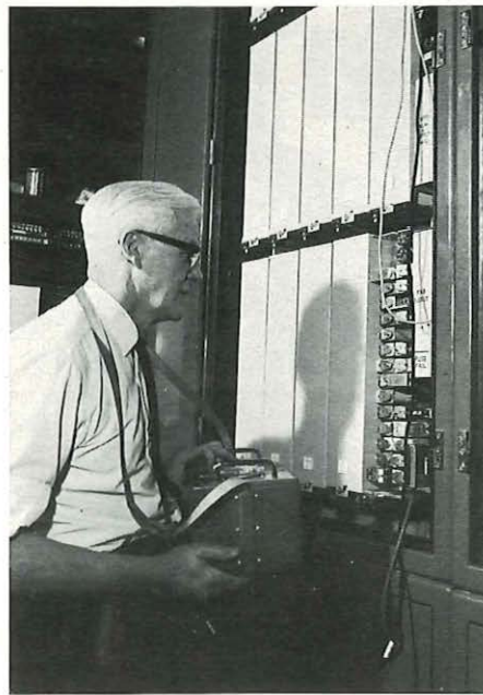
Above: Testing the relays on one of the first PATXs off the production line at Standard Telephones & Cables factory at New Southgate.
