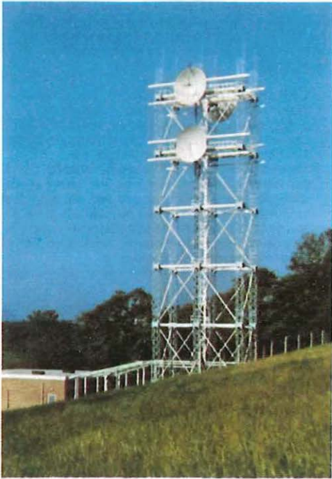
ABOVE: The new Craiglockhart Radio Station, Edinburgh, is the first to be equipped with the Tower No. 5A, developed by Post Office engineers. These towers are made from a small number of interchangeable piece parts which are assembled in a variety of configurations to form structures suited to the differing requirements at each station.
