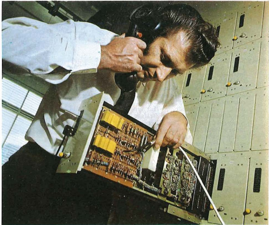
A technical officer tests one of the supervisory relay sets at the TXE 2 electronic exchange at Odiham Hants. This system is being used for almost all new small-to-medium exchanges.
