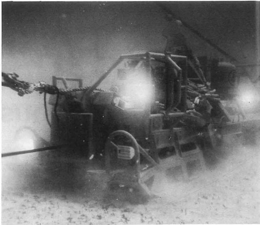
Underwater lights pierce the dark depths as the AT&T Company's plough crawls along the seabed burying a cable as it goes.
