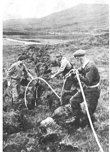
the moor to keep it safely away from extensive roadworks that were going on nearby. RIGHT: Field staff manoeuvre the cable in the open moorland trench.
