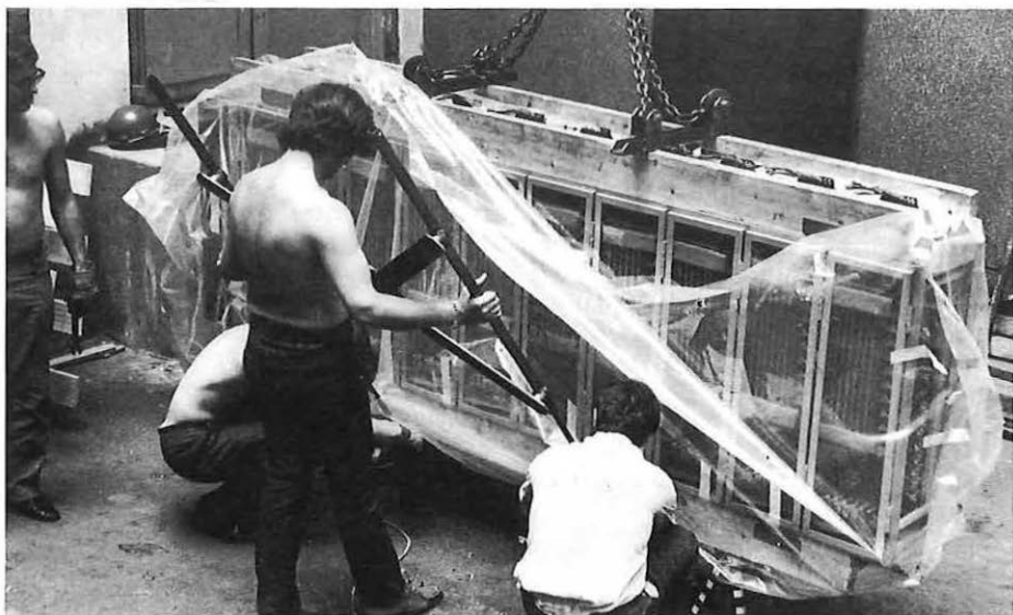
Attaching the steel framework which was used to hoist the equipment to the apparatus room at Wood Street.
