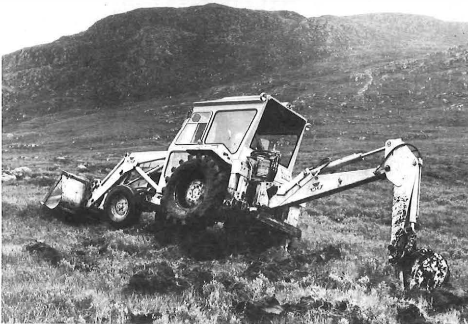
LEFT: Even this trenching machine has difficulty negotiating rough Highland moorland during the laying of the Inverness-Ullapool-Gairloch coaxial cable. This stretch was laid across
