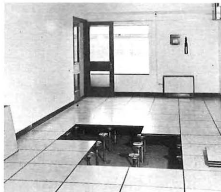
The raised false floor in the main distribution frame room at Toddington with some of the covers removed to show the void in which cables are connected.
