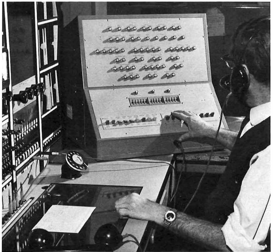
A prototype of the control console in use at Truro. The results of the tests are indicated on the lamp display unit.
