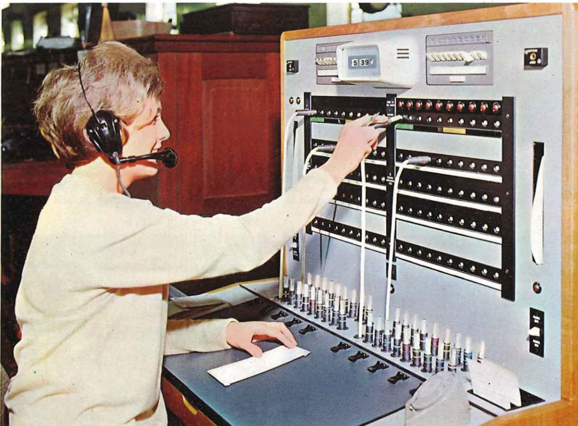
The manual switchboard at Telephone House, Birmingham, specially developed for the Datel 48K trial. Other switchboards are in London and Manchester.
