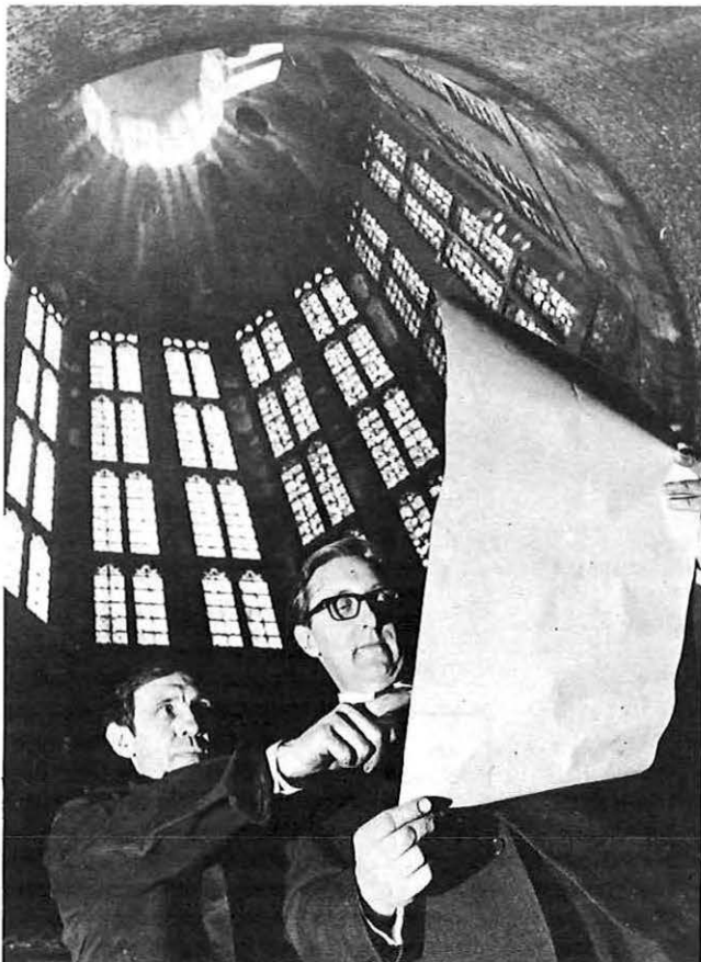
Engineers check on the cable layout at the Palace of Westminster where installation work on part of the Whitehall scheme has already started.
