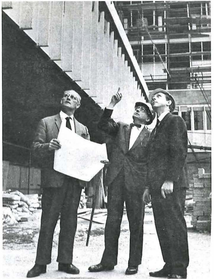
London Telecomms Region uses CPM techniques for all major projects, including the South Bank (Rampart) outgoing trunk unit. Pictured on site are (from left): Mr. T. J. Beningfield, Clerk of Works MPBW, Mr. A. C. Walter, LTR Engineering Accommodation and Mr. J. Scott of the CPM team.
