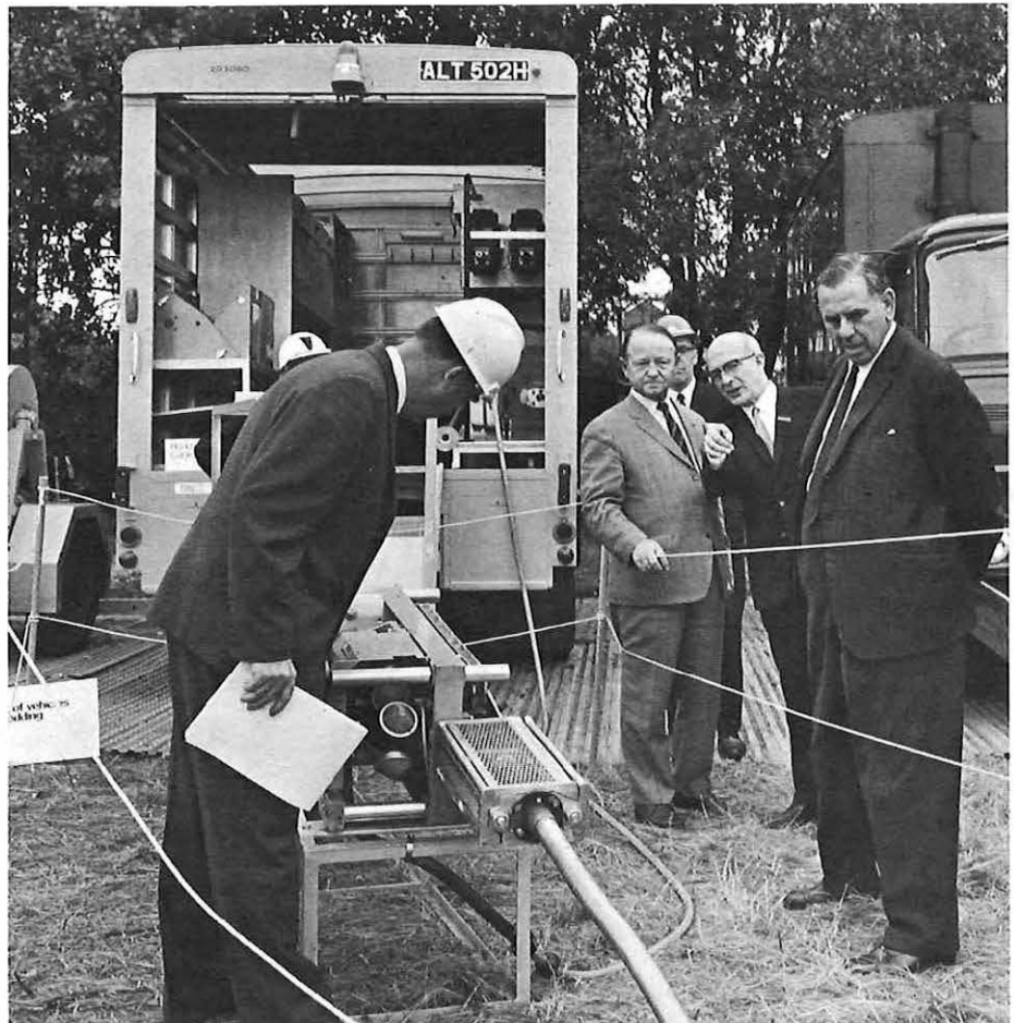
Staff Engineer Mr. A. C. Croisdale points out details of the rodding and light cabling equipment to Lord Hall, Chairman of the Post Office Board. With them (right) is Mr. A. W. C. Ryland, Deputy Chairman and Chief Executive. The rod pushing device has been taken out of the vehicle for display.
