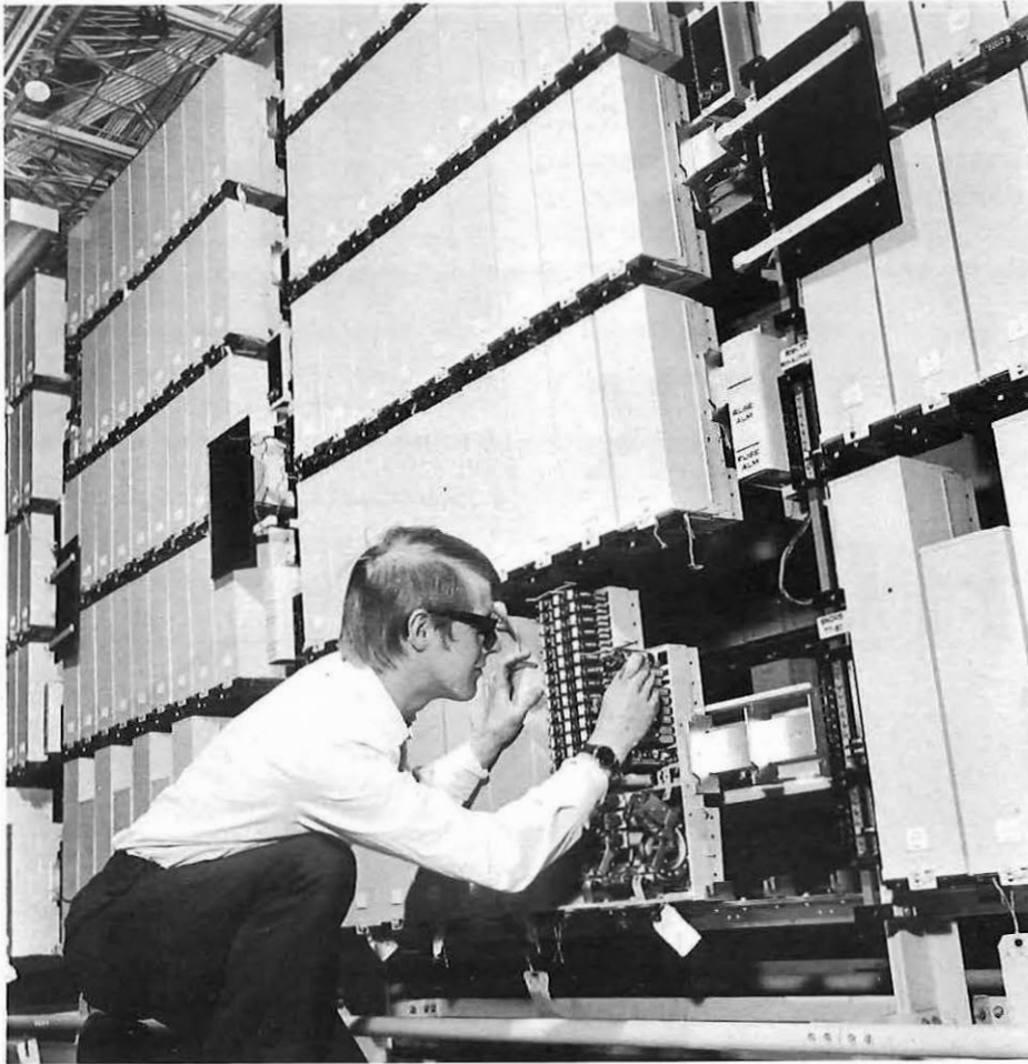
A check is made on a position sender during installation of the Croydon Cordless Switchboard.
