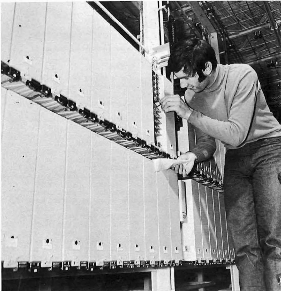
An engineer tests a queue relay set.
