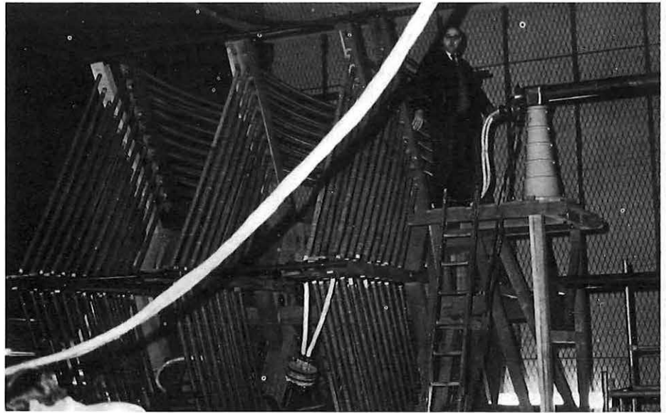
Below: The interior of the new coil room showing the main aerial tuning inductor.
