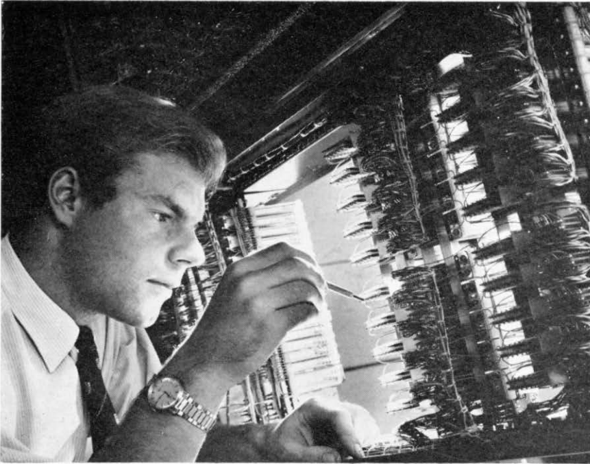
An STC engineer checks one of the contacts on a multiple relay of a crossbar exchange.
