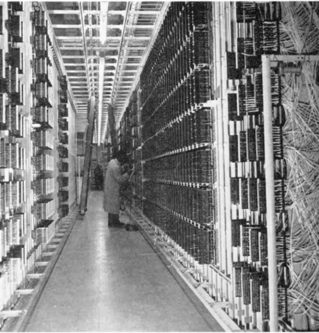
These are the two main distribution frames which serve the building. They extend to 300 verticals and are among the biggest of their kind in Britain.
