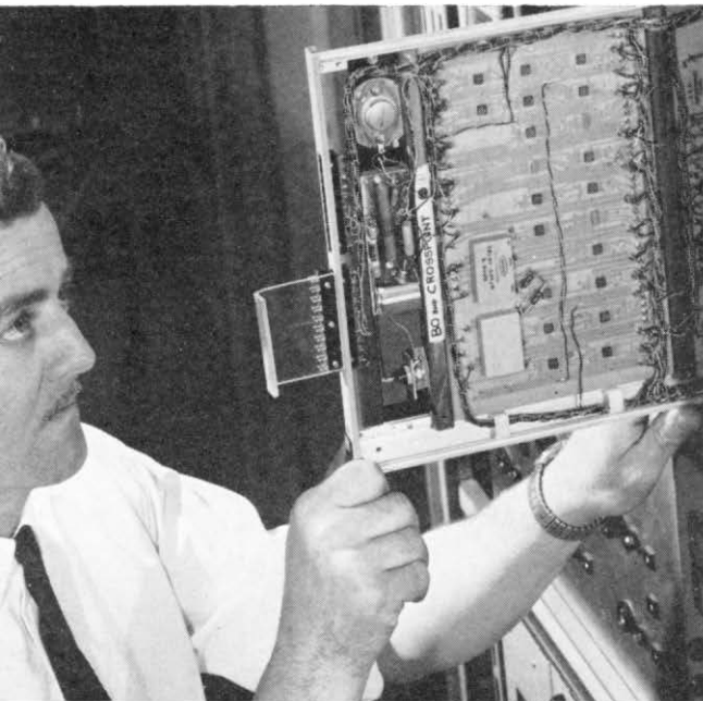
Technical Officer Mr. D. Weedon inserts a switch unit into the new PCM system at Empress.
