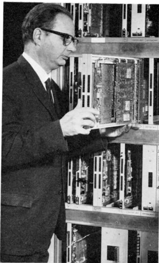
Staff Engineer Mr. W. Duerdoth, leader of the Dollis Hill team, examines a plug-in unit on an A rack of the new experimental exchange.
