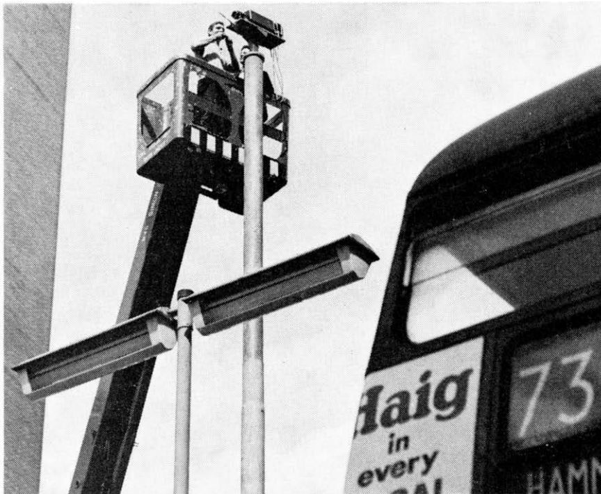
Working from a mobile tower, workmen repair a camera 40 feet above the swirling Knightsbridge traffic.
