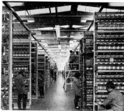
A view of the vast rack wiring sections in the new factory at Kirkcaldy.
