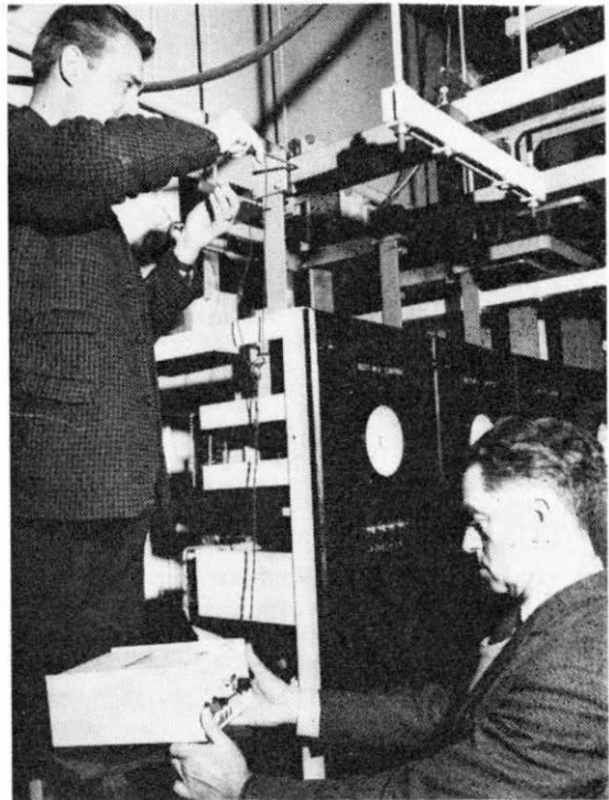
Mr. N. Purseglove, a trainee technician improver, adjusts the voltage relay which controls the busbar voltage. The operation of the power plant depends entirely on the correct setting.
