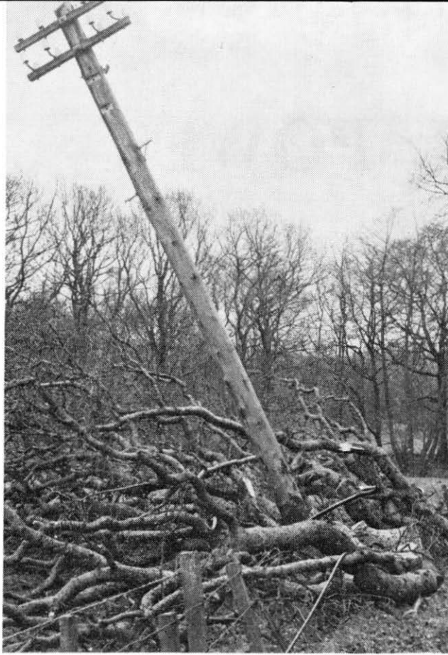
On the road from Balmaha to Rowardennan a pole sways drunkenly, its cable torn apart.
