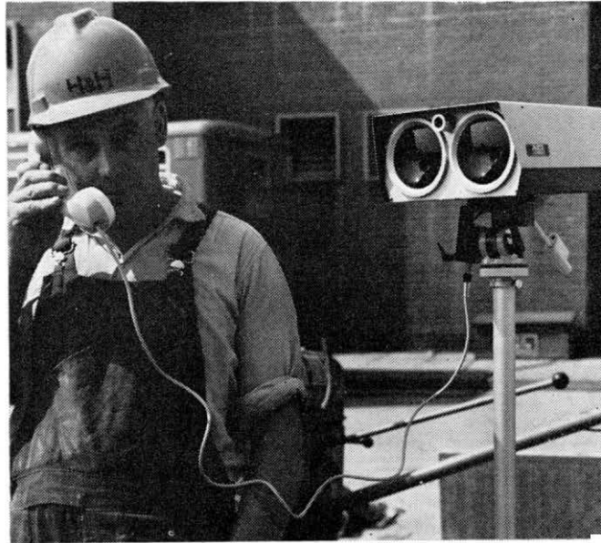
The new equipment in use on a building site. It has a range of up to one mile and is simple to use.
