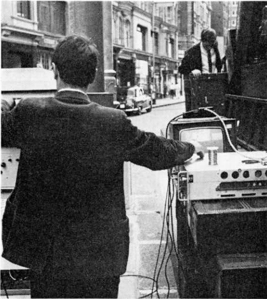
An installation team checks the camera equipment at a busy road junction in Knightsbridge—one of the eight camera positions in West London.
