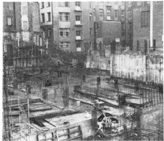
The concrete reinforcing rods rise and Dial House begins to take shape. It will be completed and ready for service by autumn, 1970.
