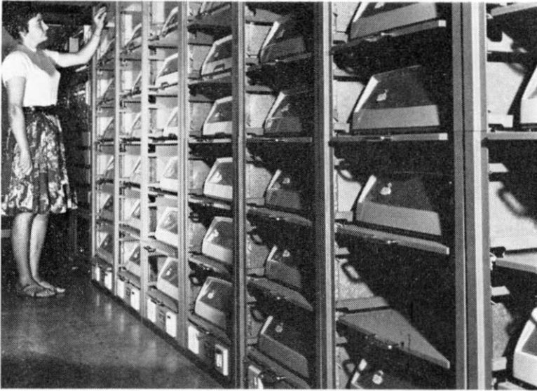
Rack-mounted Datel 200 modems being used with automatic answering facilities at a multi-access computer installation.
