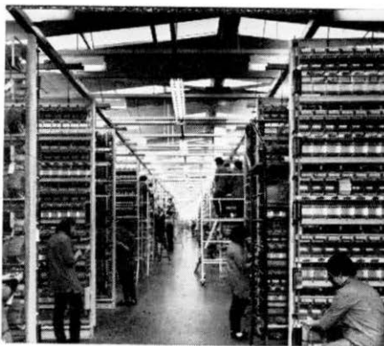
A view of the vast rack wiring sections in the new factory at Kirkcaldy.
