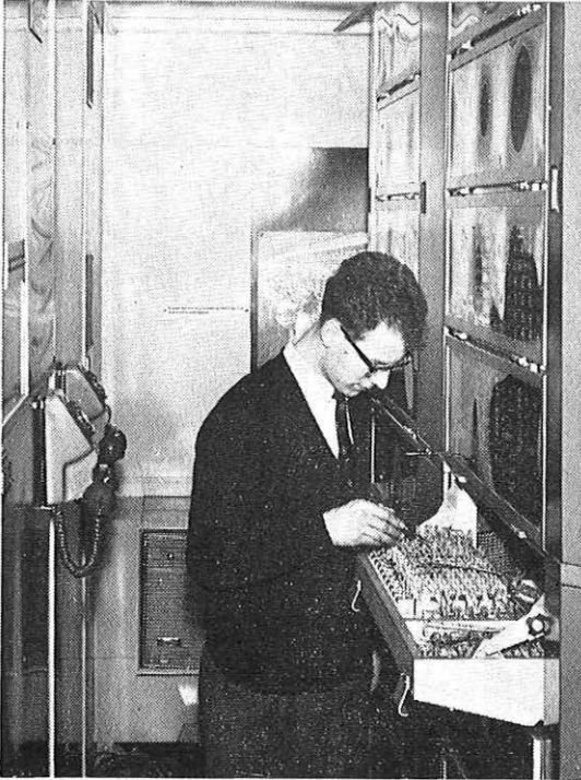
An engineer examines and tests part of a 5005 crossbar exchange, similar to that which will be installed at the new Wood Street Centre.
