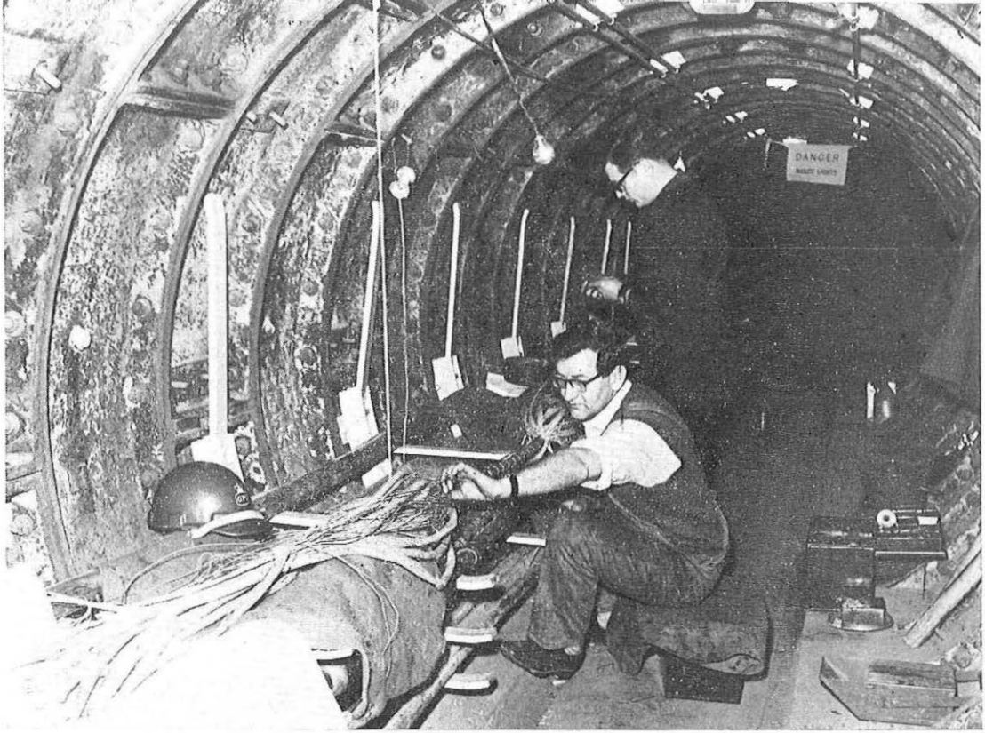
LTR technicians joining cables in one of the seven-ft diameter tunnels beneath Oxford Circus. Each tunnel is about 300 yards long. All tunnel shafts and manholes are electrically lit and ventilated.
