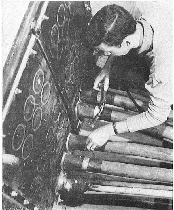
A joiner plumbing a new cable into an old-style duct seal. Note the lead tubes.
