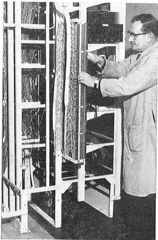
Technician 11A Mr. H Radford blocks off the manual switchboard at Ambergate before the new electronic exchange is brought into use.
