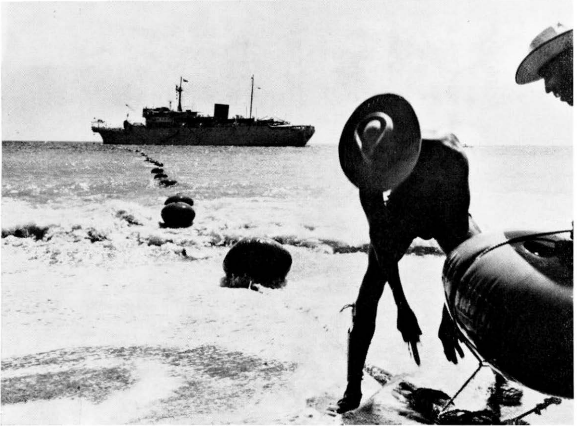
Venezuelan workmen remove a float from the cable after bringing it ashore at Maiquetia. Offshore lies Alert
