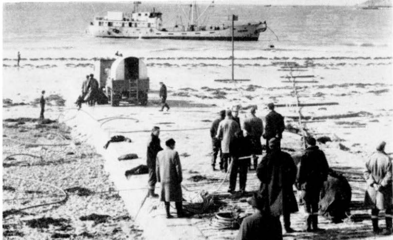
The Dutch cable ship Poolster lies off St. Helier as the shore-end cable is landed and work begins to link it to the repeater station.
