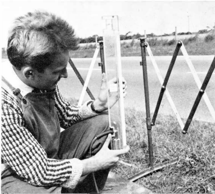
Checking cable pressure with the Post Office standard manometer No. 1B. The column of mercury adjacent to the scale on the right-hand side of the instrument indicates the cable pressure directly in lbs per square inch above normal atmospheric pressure.
