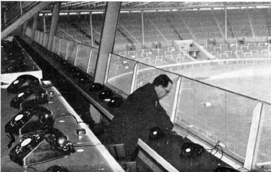
GPO Technician Albert Roper sets up and tests some of the 240 telephones which have been installed in the Press Box at Wembley Stadium.
