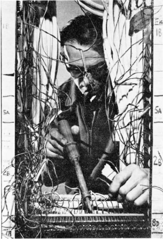
Above: Most of the World Cup traffic will pass through three switching racks at the International Programme Switching Centre at Faraday Building, London. Here, Mr. William Syms solders some of the 48,000 connections.
