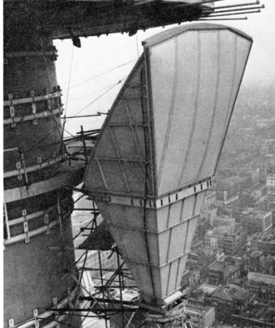
A close-up of a microwave horn aerial at the Post Office Tower in London, focal point of the nation-wide radio relay system which is being extended throughout the country.
