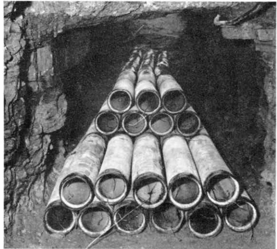
An 18-way formation of the new earthenware duct. The formation can be changed to negotiate obstacles and thus often save costly methods of construction.
