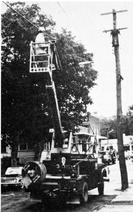
The Engineering Department is carrying out trials with this American construction vehicle which can erect aerial cables three or four times faster than any other method.
