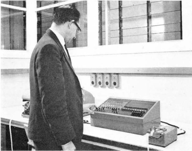
AEE A. R. Lawrence, of the Main Lines Development and Maintenance Branch, operates the main control board of the new ATME equipment. Note the tape-reader (right).
