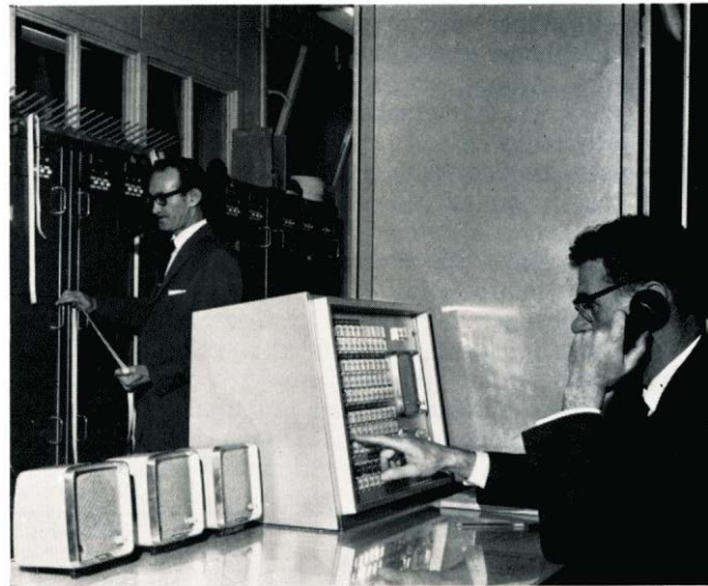
The new push-button controlled switching equipment (foreground) recently installed in the London centre and (background) part of the teleprinter torn-tape relaying equipment which is soon to be replaced by an automatic computer system.
