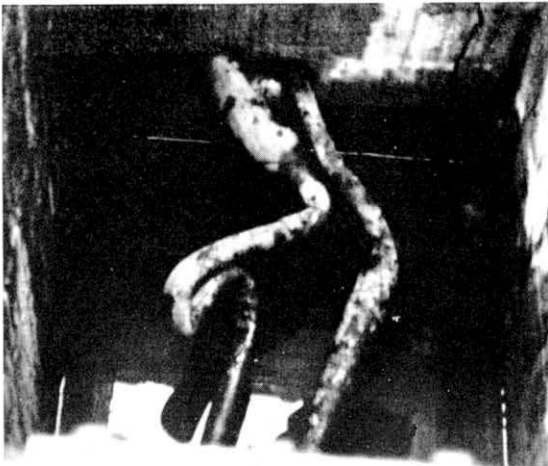
Above: A lead-sheathed trunk cable distorted by creepage caused by traffic vibration. Right: An example of the effects of corrosion.
