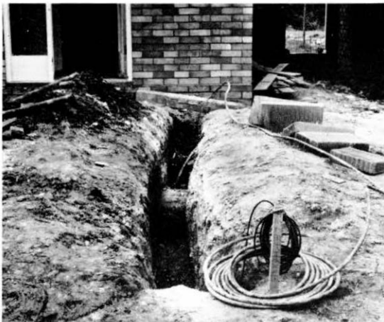
A lead water pipe and an armoured polythene telephone cable are being led into a house under construction through a common trench.
