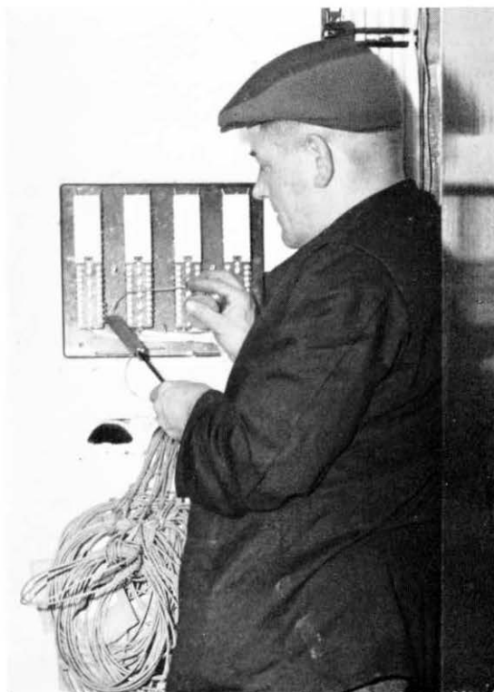
Post Office staff at work on the Piccadilly Plaza Project. Left: T2A J. Ball strips insulation on a riser cable before jointing. Right (above): T2B C. Slater examines wiring on a main distribution frame; (below): TO W. Helliwell tests a riser.
