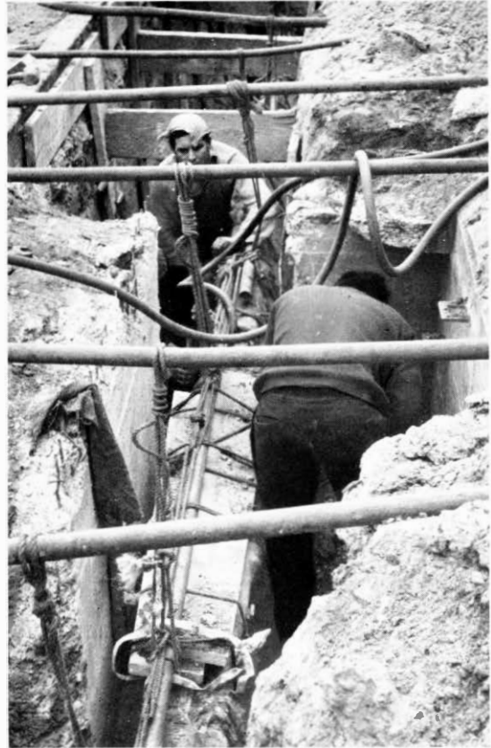
As the underground trunk cable system grows jointing chambers have to be re-constructed.
