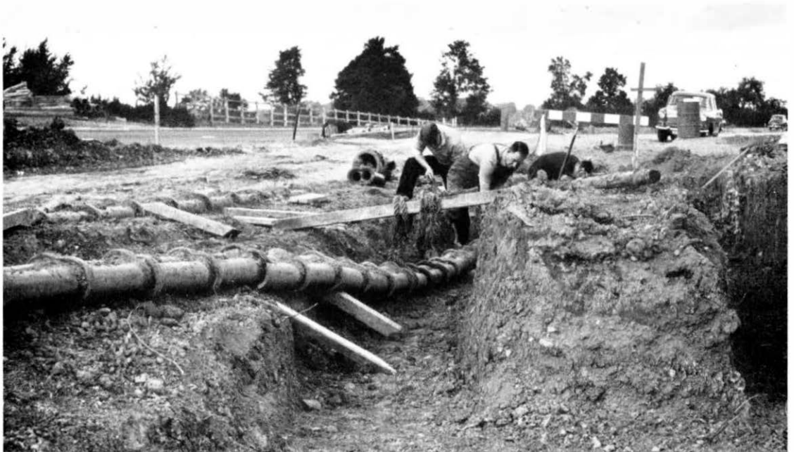
Road widening schemes often mean the costly and time-consuming job of digging up duct tracks and slewing them into new trenches. Carrying out this operation can result in damage to cables.
