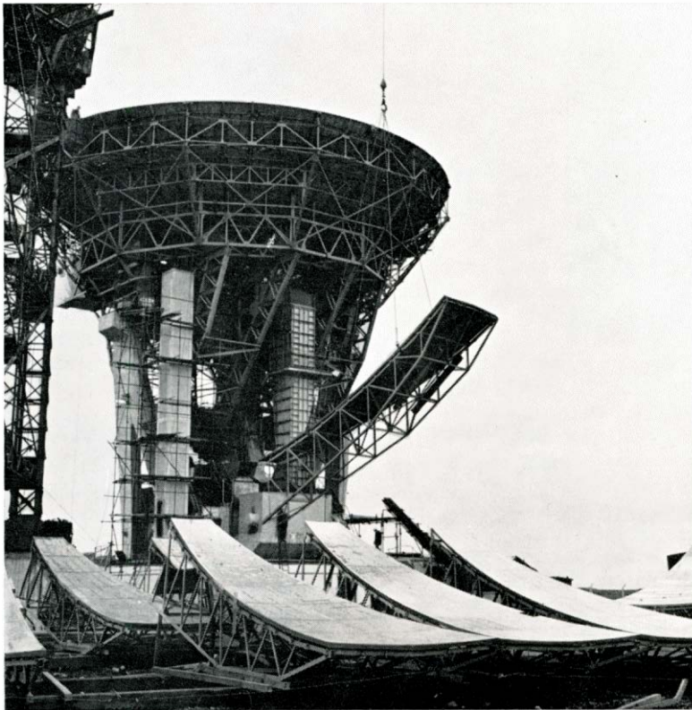
One of the 30-ft long petals for the new parabolic dish aerial is hoisted into place.
