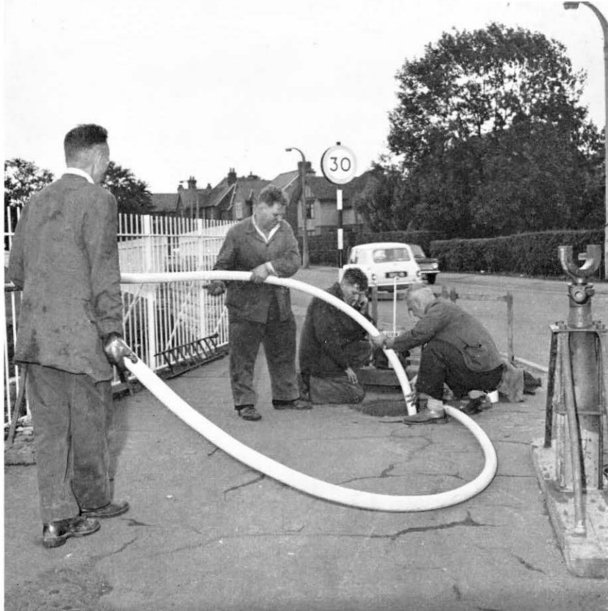
While one man sends instructions to the winch, the last loop of a polythene cable is eased into a manhole. This cable will provide telephone service for 2,000 subscribers.
