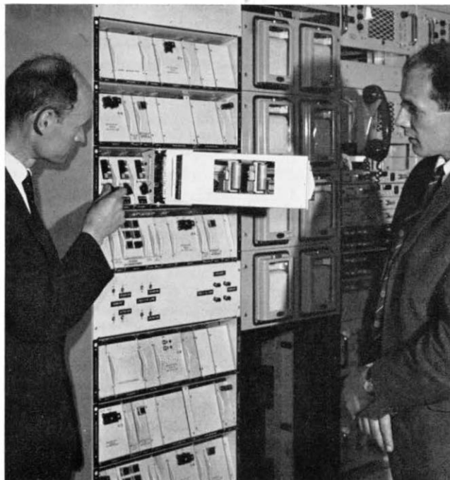
A partially-equipped new double-depth type 62 rack with a card in its hinged outrigger, showing sloping card fronts.
