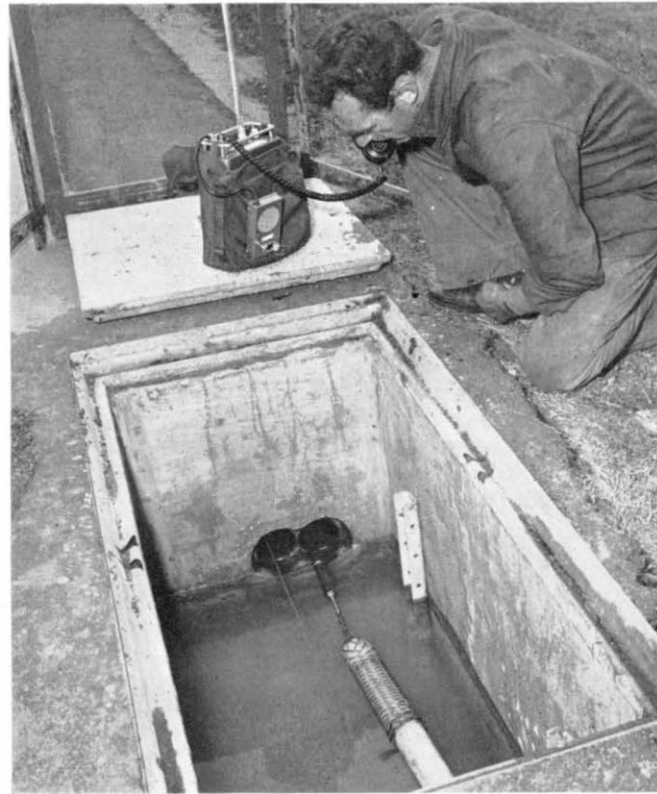
As the cable end passes through an intermediate jointing box a member of the cabling gang reports progress.
