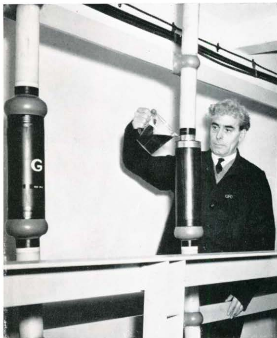
Liquid epoxis resin is poured into the open end of the sleeve of a vertical air block in a large size polythene insulated and polythene sheathed cable.
