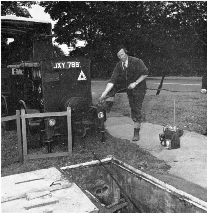
Waiting at the winch for a call over the transceiver to begin cabling. The transceiver shown here is the No. 1A, the first portable set to be used by non-radio Post Office staff on external work.
