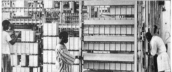
Automatic telephone exchange equipment at Ibadan, Nigeria
