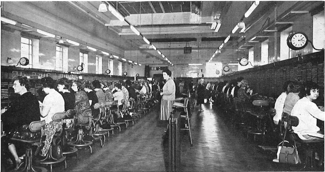
The incoming and inquiry positions on the switchboard in Telephone House today.
