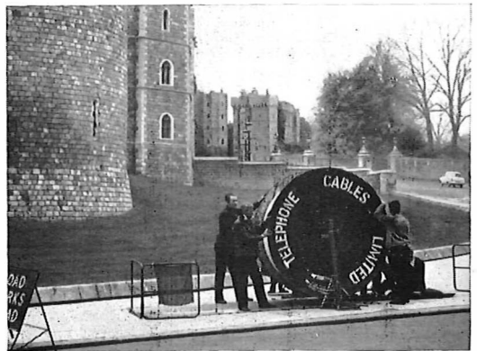
T.C.L. moisture barrier cable at Windsor Castle
