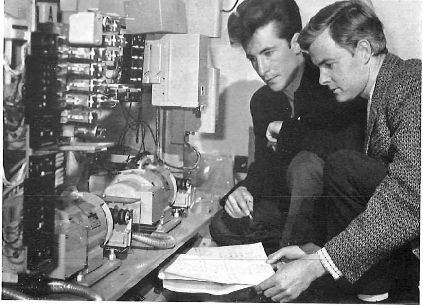
Technical Officers W. H. Tollerton and W. R. McCusker, both from Belfast Area, test the ringer bay at the main Harwell Exchange. Right (below): Technician T. Kirk adjusts the MDF "jumpers".
