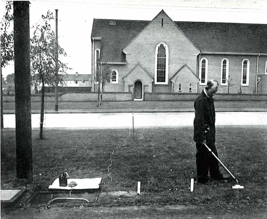
THE NEW. Locating an underground cable with the new apparatus. Note the transistorised oscillator and earth spike at the joint box and the miniature search coil.
