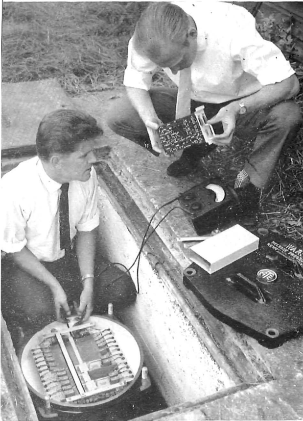
Two Automatic Telephone and Electric Company's engineers installing one of the PCM repeaters for the trial between Reading and Marlow. When fully equipped, 12 24-channel, bi-directional repeaters are accommodated. Picture: Courtesy ATE.
