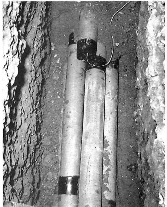
Part of the six-way nest of the new duct built in a pyramid formation under a suburban roadway. The result of this trial so far is very satisfactory.
