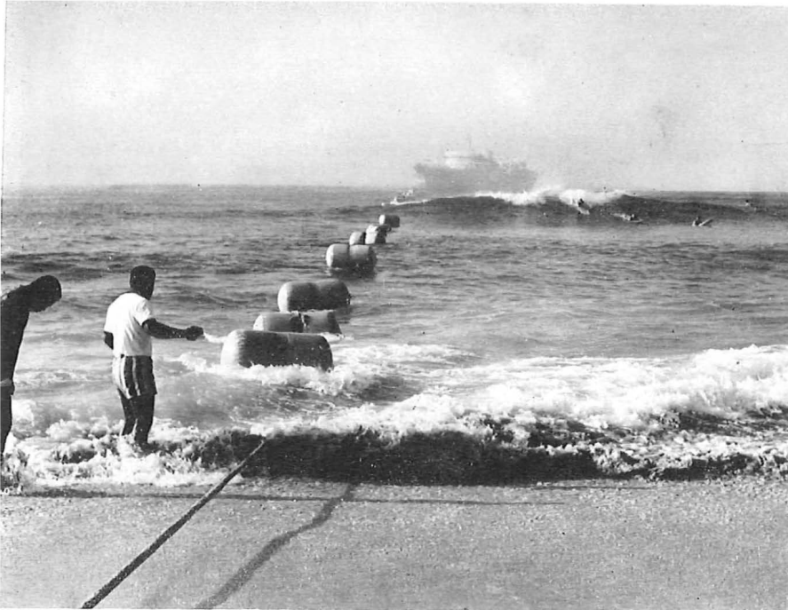
The shore-end of the Sydney to Auckland section of the COMPAC Cable is floated ashore at Bondi Beach from the Cable and Wireless Company's cable-ship Retriever . SEACOM, the third stage in the Commonwealth Cable Scheme is now under way.
