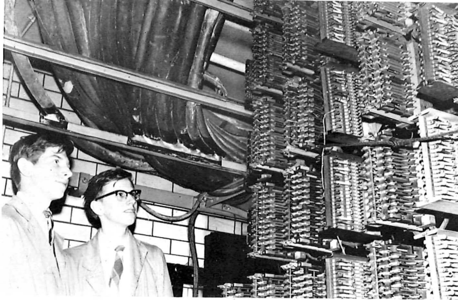
Young engineers examine the overhead feed of the underground cables into the main distribution frame verticals. These cables rise to a height of 50 feet.
