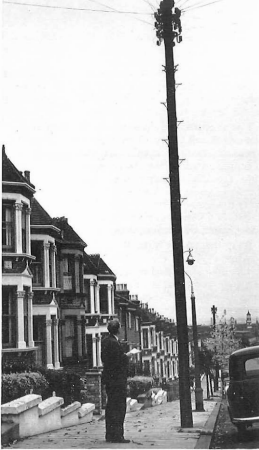
Technical Officer L. H. Fenwick checks the number of subscribers' lines and the size of the multiple cable at a distribution pole in Waller Road, New Cross, London.
