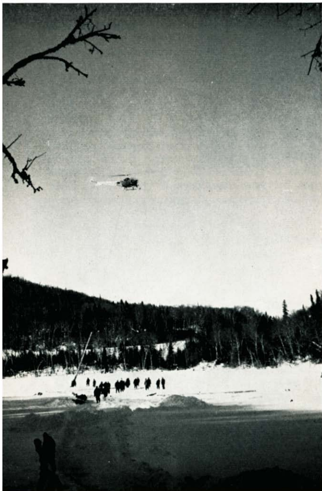
A helicopter lifts in a 40-ft long power-line pole at Marathon, Ontario, to supply electric power for a remote microwave tower—one of 136 which are being erected across Canada.
