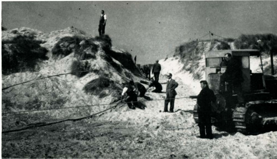
Left: Post Office staff from Norwich Area handling a cable ashore. Above: Winching in the sea earth cables. The cables were hauled up the beach and through a trench in the sand-dunes to the anchorage manhole.
