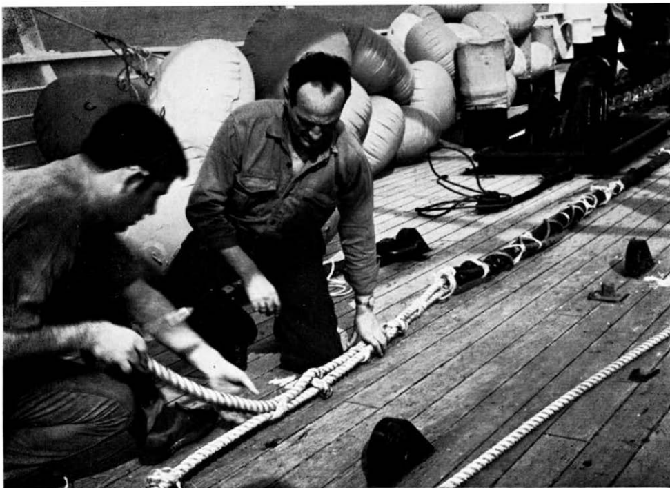
On the foredeck of HMTS Alert , the cable end is secured to a tow rope before the shore-end cable is taken ashore.
